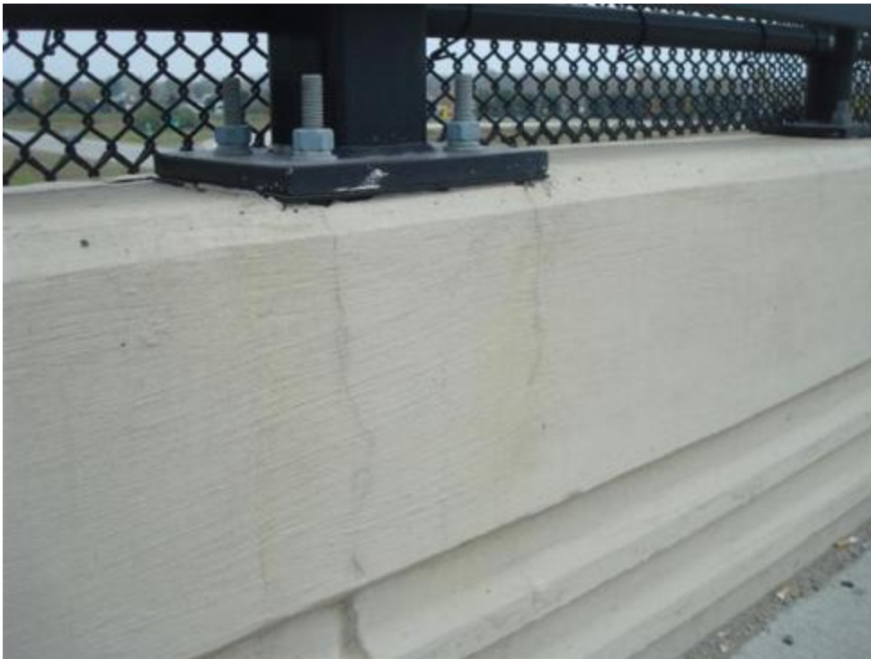
Figure 76. Cracking in barrier, at railing connection (typical)
