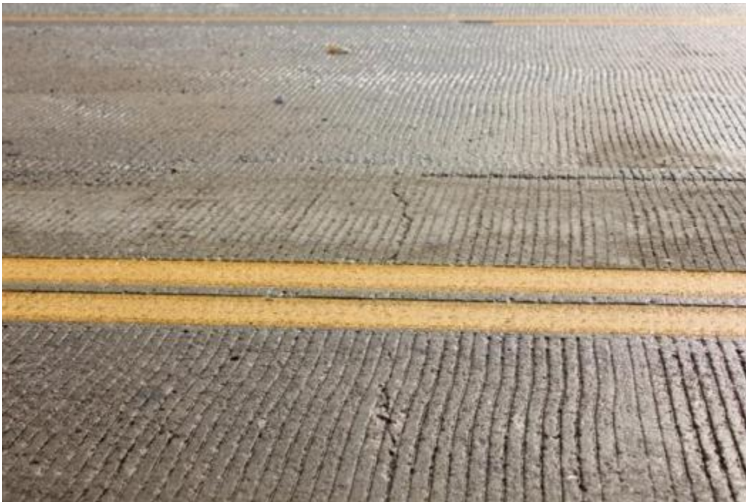
Figure 138. Transverse cracking in the middle of the bridge
