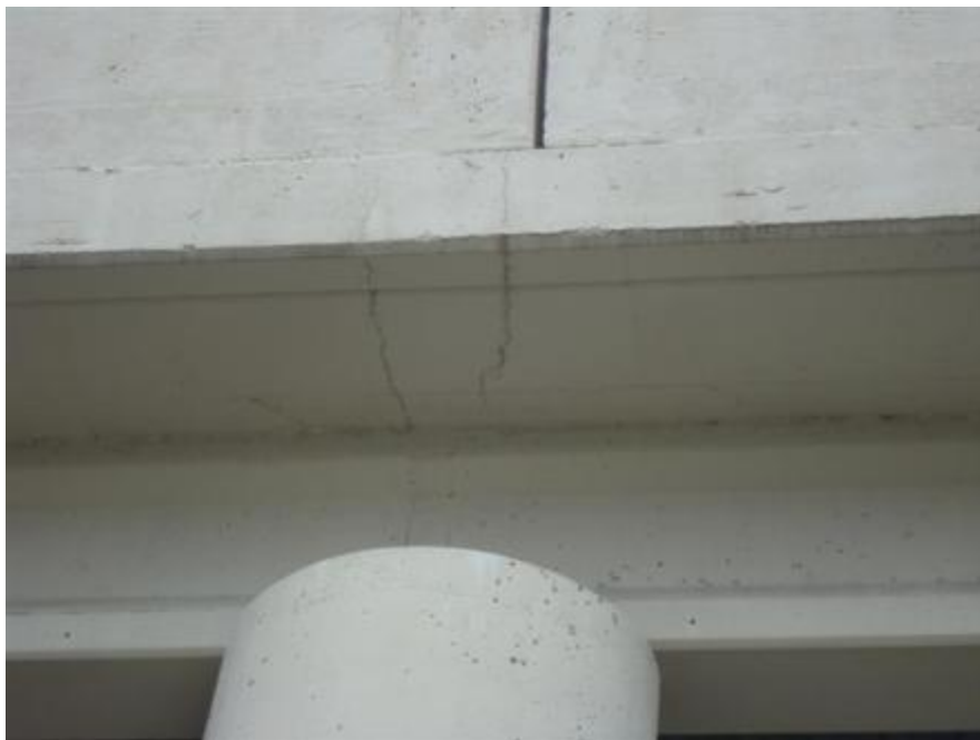
Figure 30. Cracking on underside of deck, by the pier area
