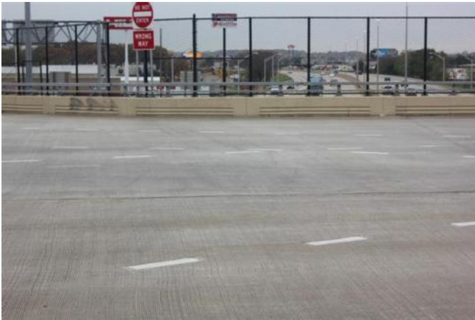
Figure 113. Transverse cracking in bridge deck
