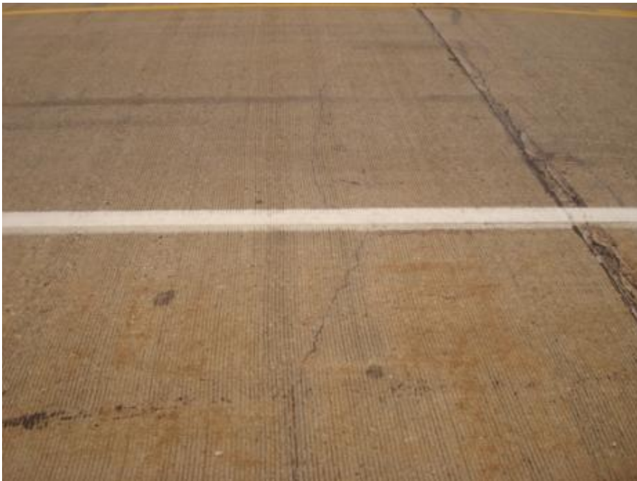
Figure 25. Transverse crack near construction joint
