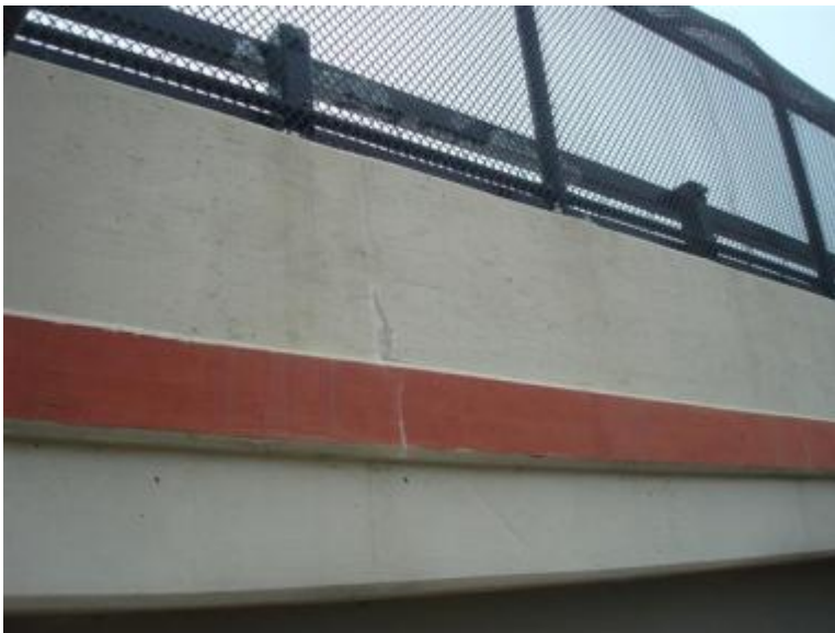
Figure 72. Cracking in outside fascia of deck and barrier
