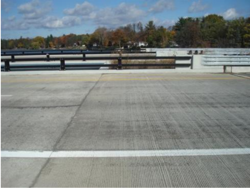
Figure 56. Longitudinal cracking in bridge deck
