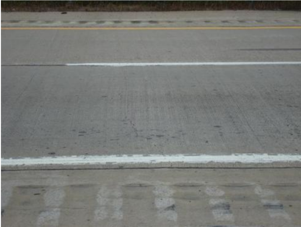
Figure 8. Cracking in approach pavement
