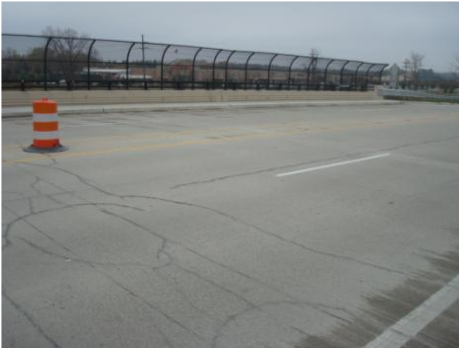
Figure 80. Transverse and longitudinal cracking
