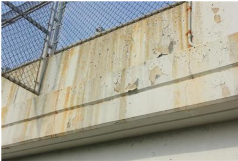
Figure 130. Deteriorated outside/fascia of the bridge
