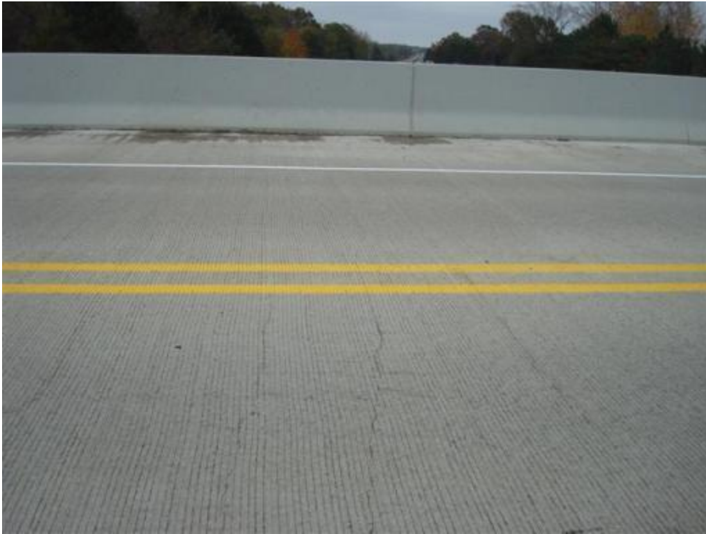
Figure 42. Transverse cracking in pier area
