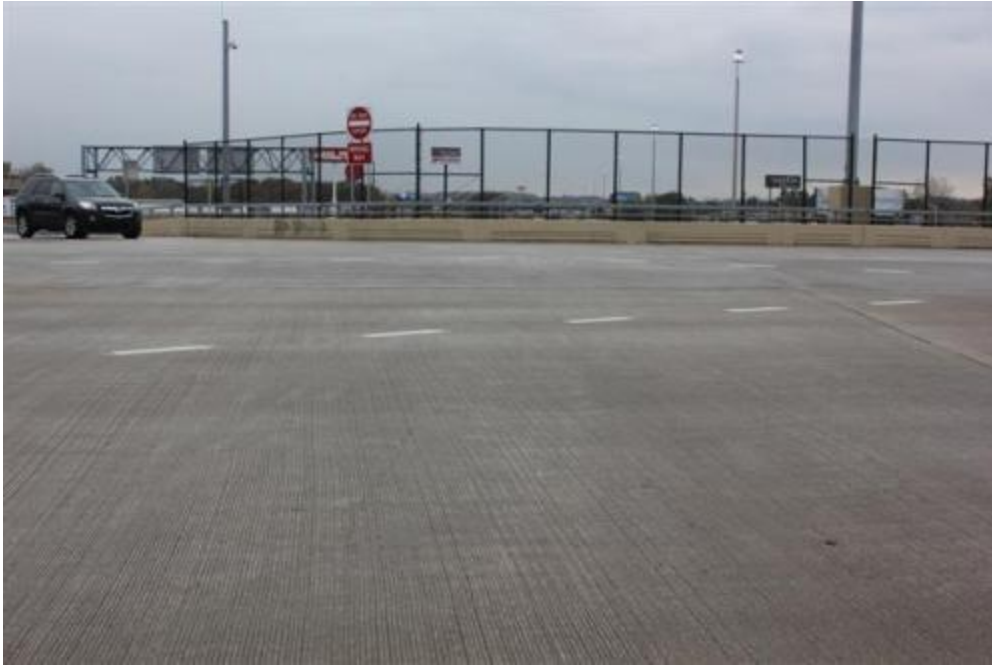
Figure 112. Transverse cracking in-between pier and abutment
