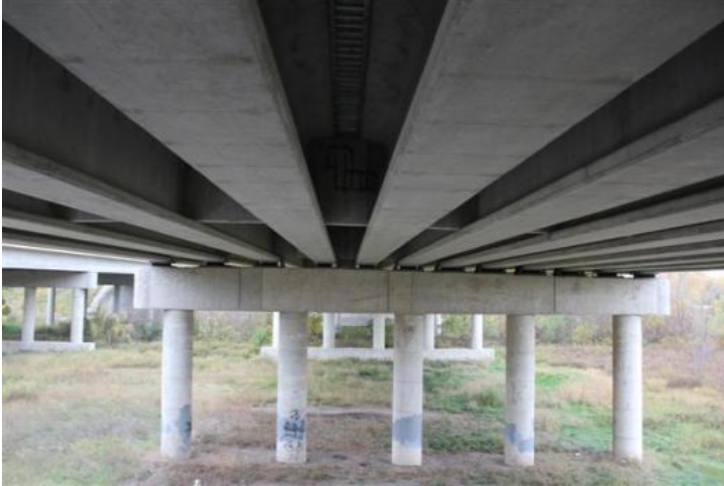
Figure 102. Bridge underside view (girder spacing is larger in the left side of the photo)
