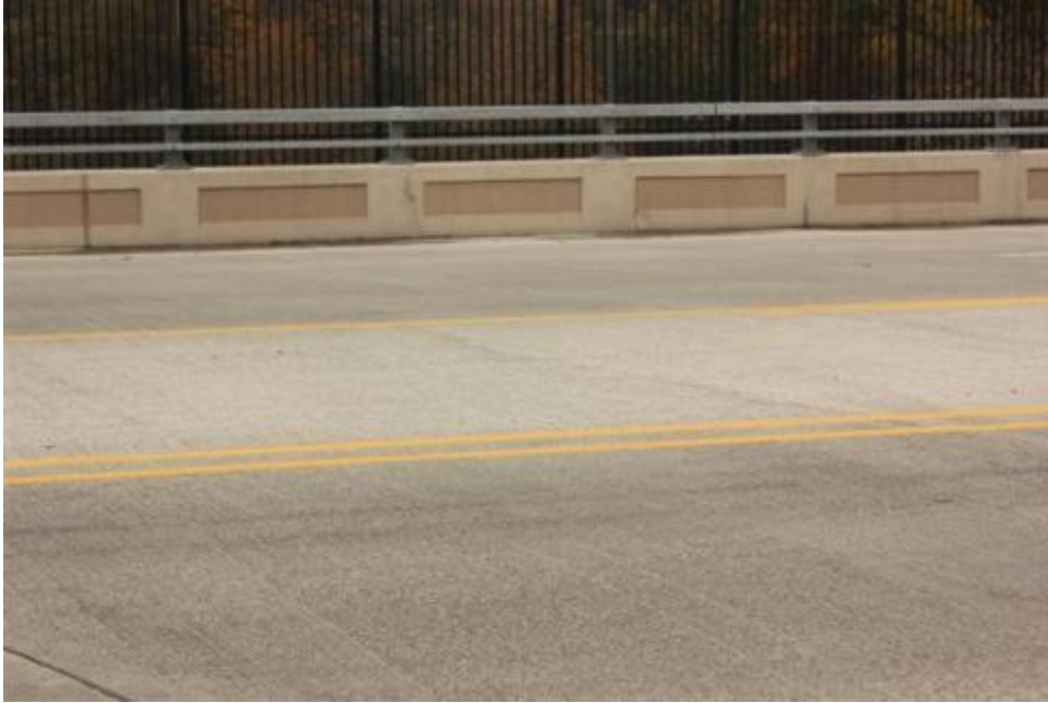
Figure 94. Cracking in barrier wall, potential transverse crack in the middle
