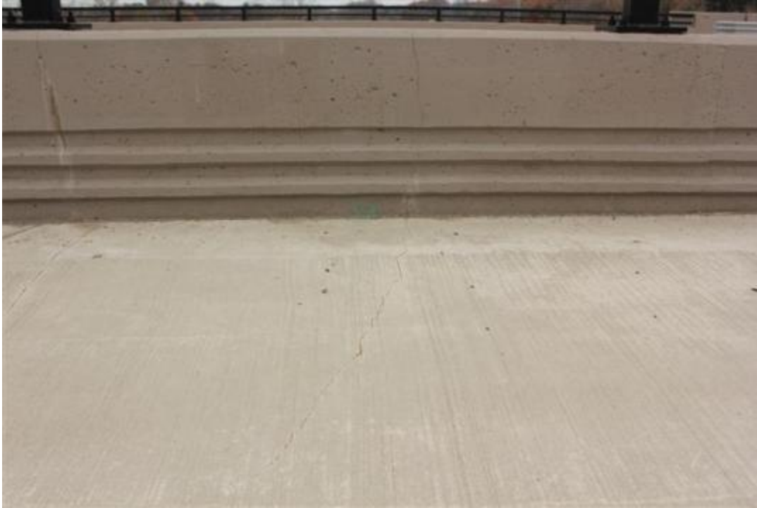
Figure 68. Transverse/vertical cracking in sidewalk and barrier wall
