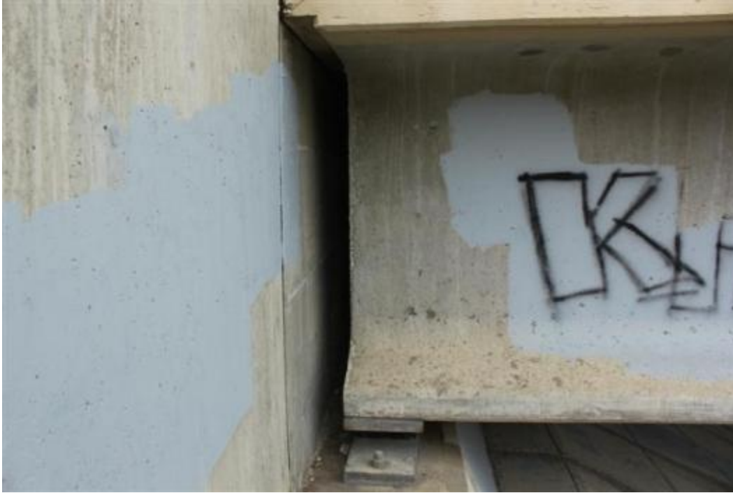
Figure 101. Non-integral abutment detail (note that beams are not cast into the abutment)
