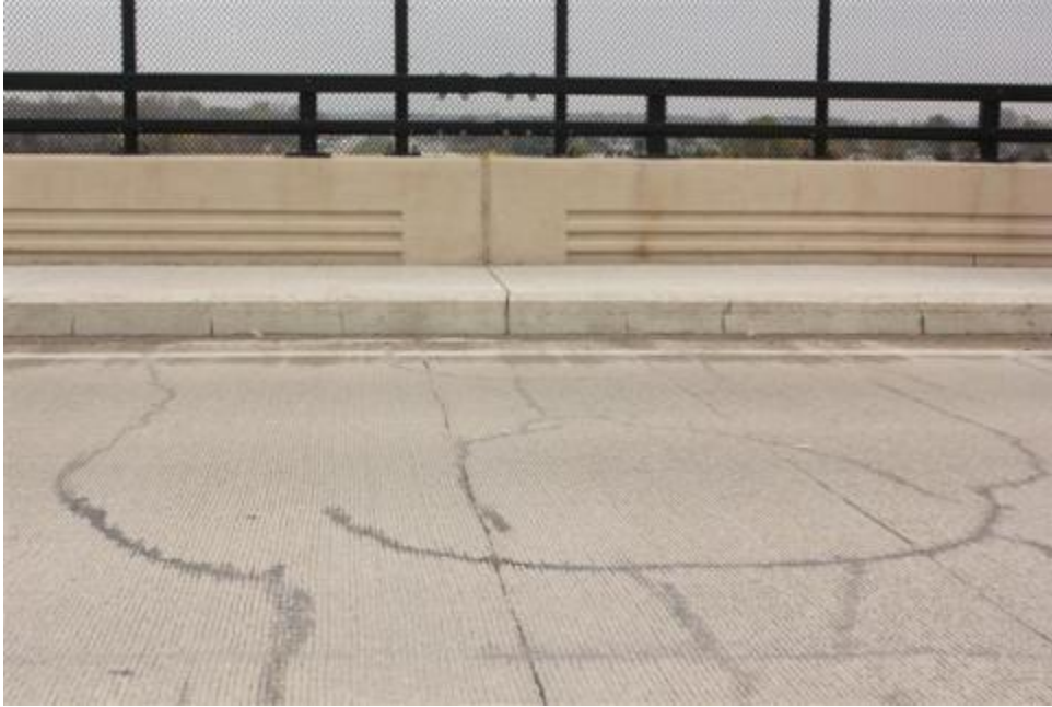
Figure 79. Transverse cracking continuing into the sidewalk
