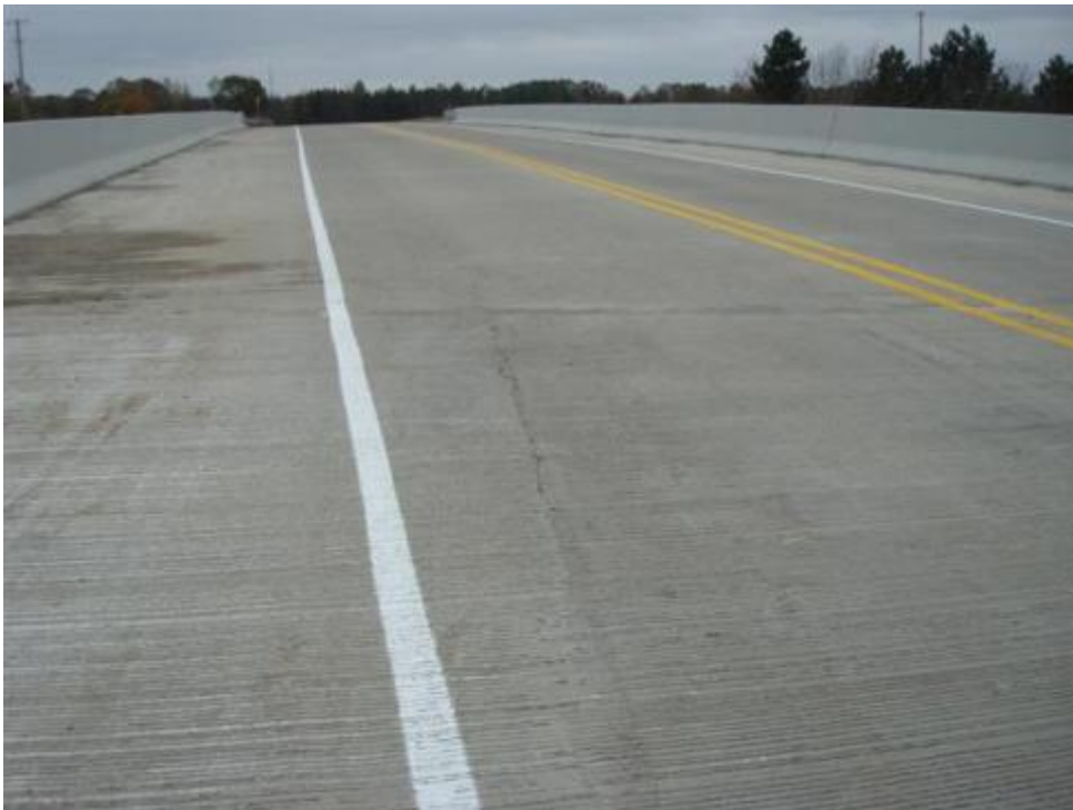
Figure 37. Longitudinal cracking in bridge surface
