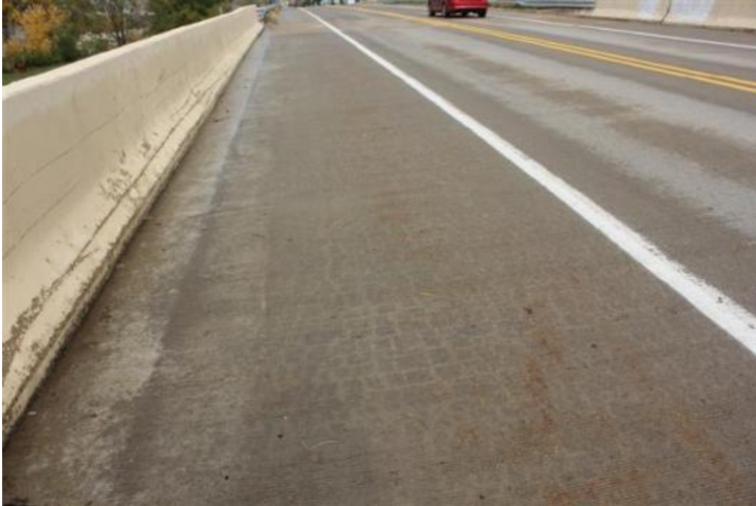
Figure 126. Random/map cracking on the shoulder
