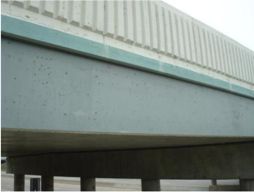
Figure 2. Cracking in deck fascia
