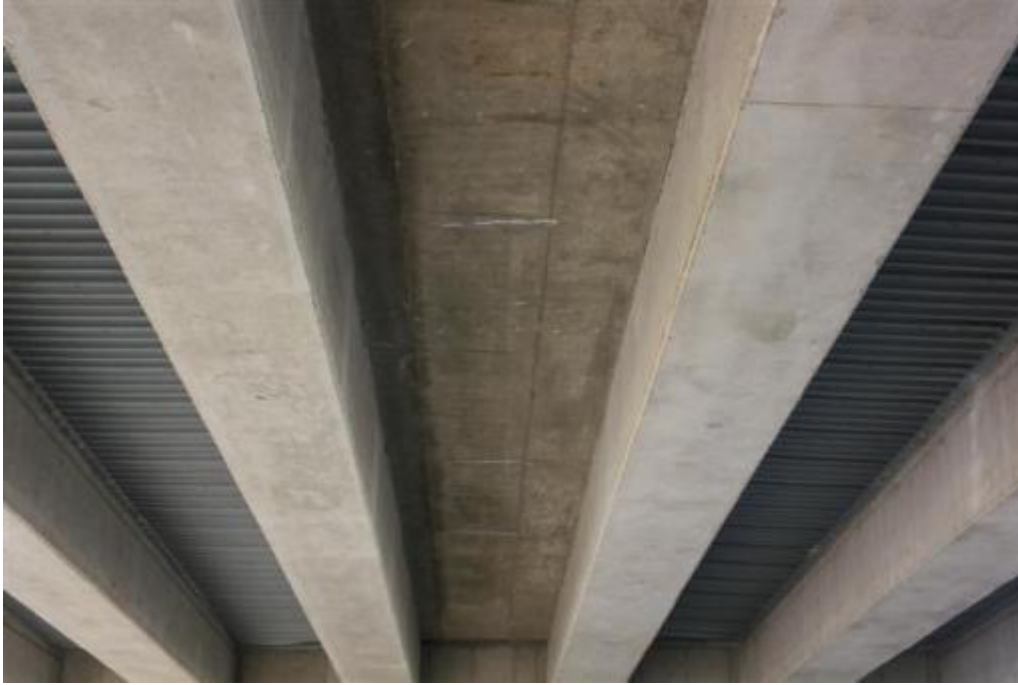
Figure 133. Transverse cracking in bridge underside
