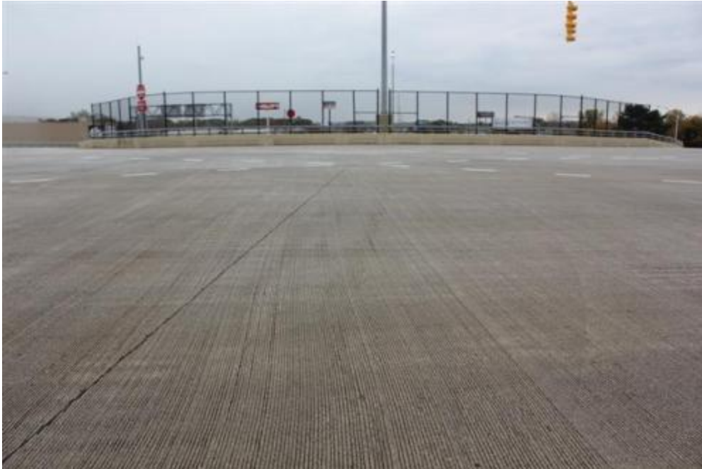
Figure 111. Transverse cracking in pier area
