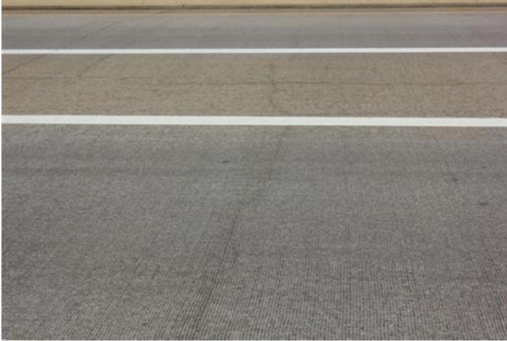
Figure 107. Transverse cracking in bridge deck
