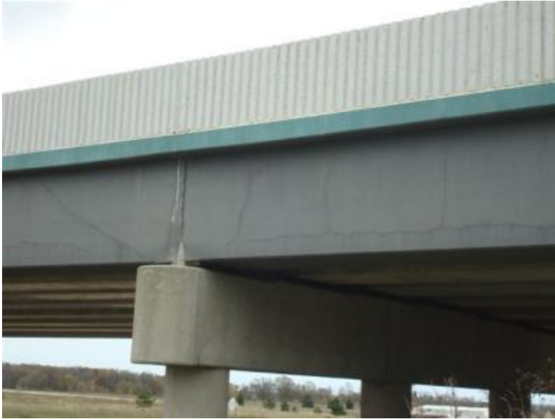
Figure 20. Cracking in beams by the pier
