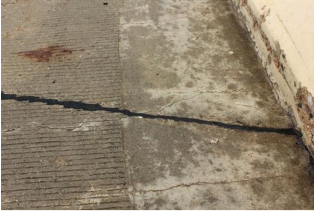
Figure 120. Transverse cracking in pier area
