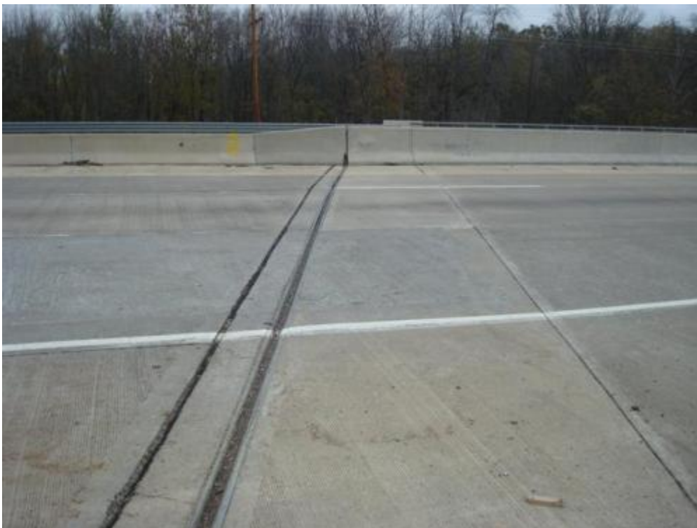
Figure 48. Bridge expansion joint and approach slab (some cracking in approach)
