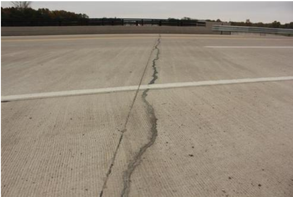
Figure 65. Large transverse crack at the abutment
