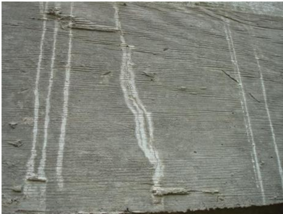
Figure 12. Cracking in deck fascia
