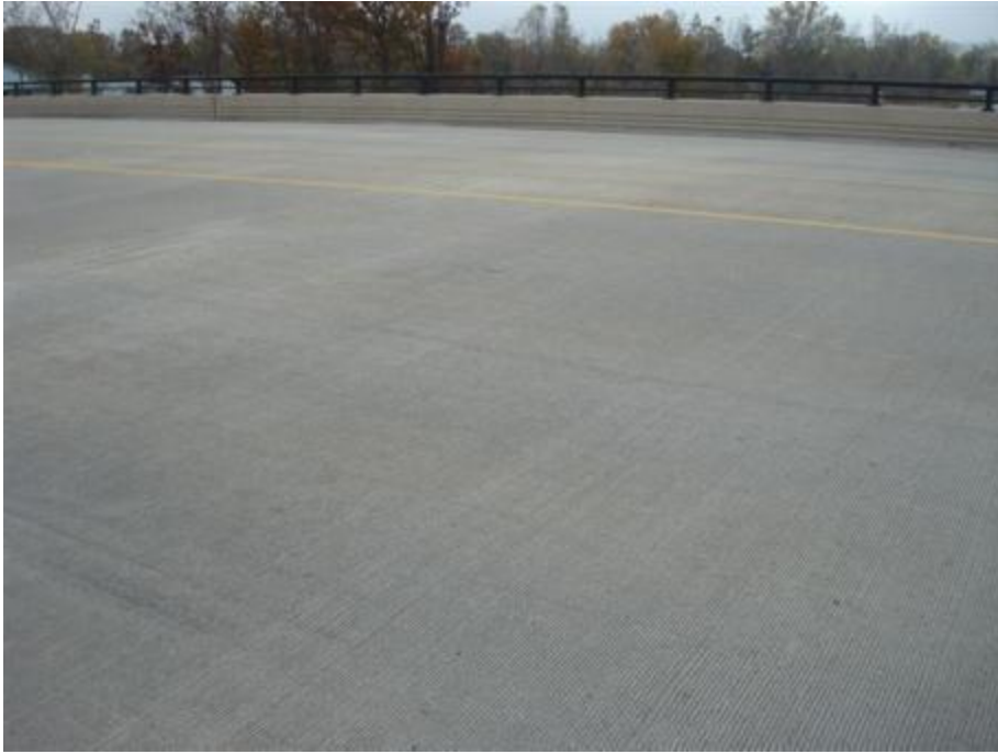
Figure 87. Longitudinal cracking in bridge surface
