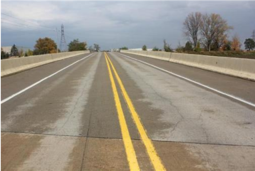
Figure 128. Longitudinal cracks running through entire deck
