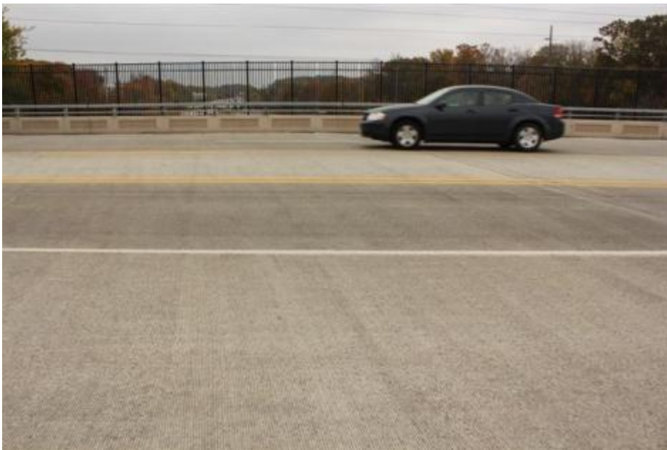
Figure 93. Possible longitudinal crack in the middle (it was not clear in the investigation whether it was a crack or roughed surface)
