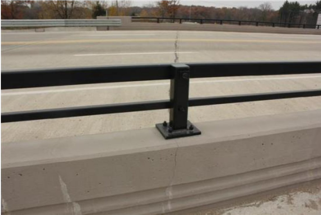
Figure 70. Transverse cracking in barrier continuing to deck surface
