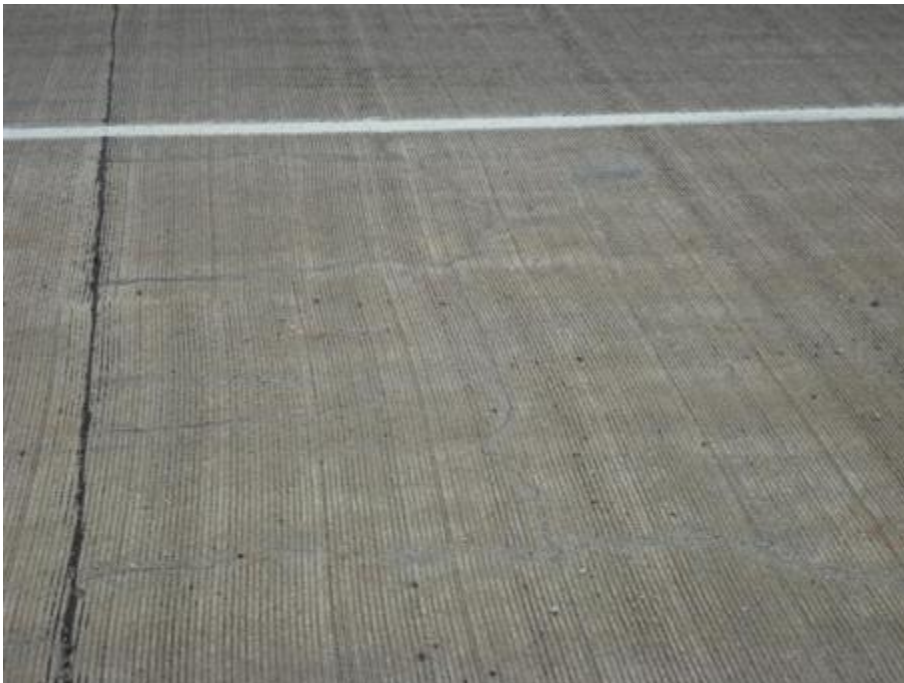
Figure 3. Longitudinal cracks in the deck surface, near the approach slab
