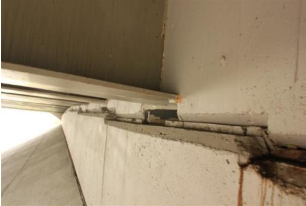
Figure 62. Bridge connection at the abutment (note that the steel girders sit on elastomeric bearings, and are cast into the abutment, similar to box-beam bridges we have seen)
