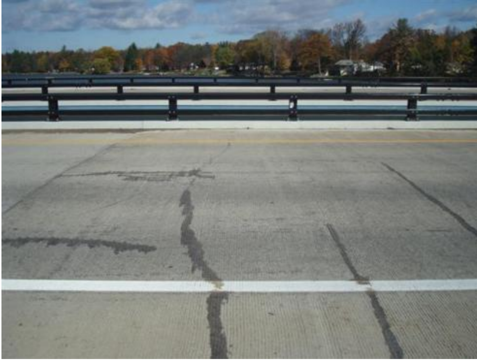
Figure 57. Transverse cracking near the first pier
