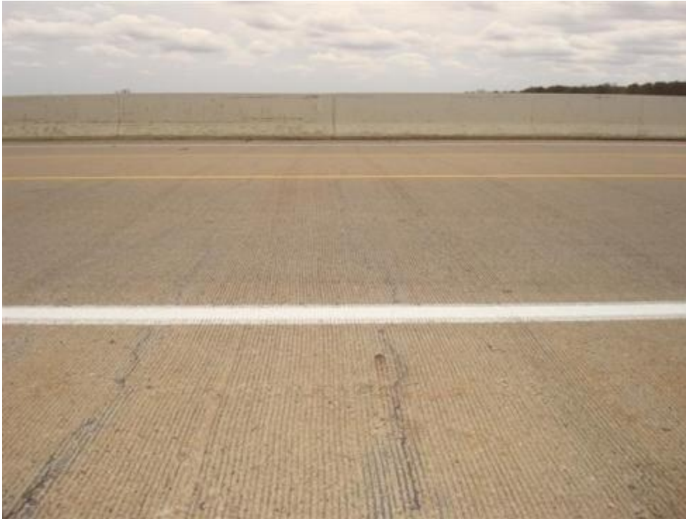
Figure 28. Transverse cracks in deck
