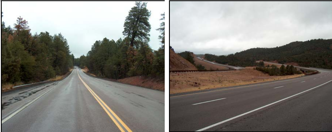
Figure 2. Existing Two-Lane Roadway, Doubtful Canyon Section (Left), Being Reconstructed into a Four-Lane Divided Highway, Preacher Canyon Section (Right).
