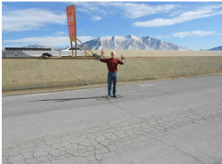
Figure 10. Photo showing cracks at one of the six locations in Figure 9.
