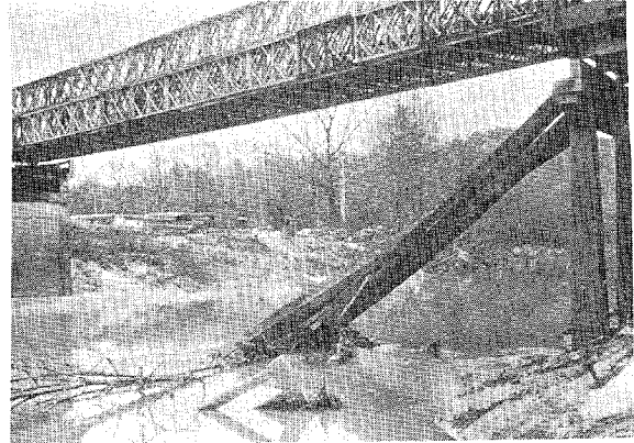
Figure 14. BRIDGE FAILURE AT SR-8 OVER BATUPAN BOGUE NEAR GRENADA, MISS.
