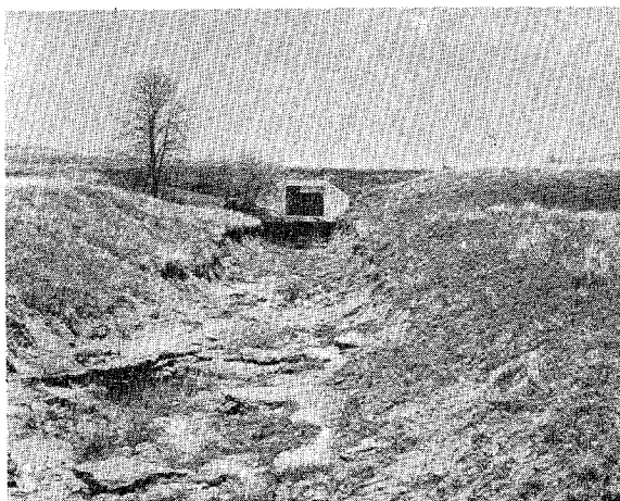
Figure 30. DEGRADATION DOWNSTREAM OF CULVERT
