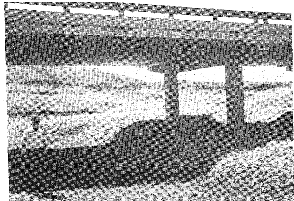
Figure 21. AGGRADATION ON BIG ELK CREEK AT I-90 IN S. DAK.
