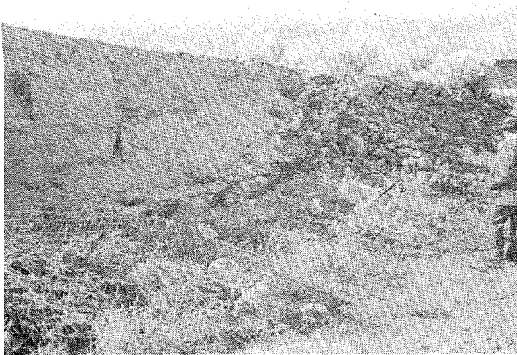
Figure 13. UNDERMINING OF BANK PROTECTION AT SR-78 NEAR VELARDE, N. M.
