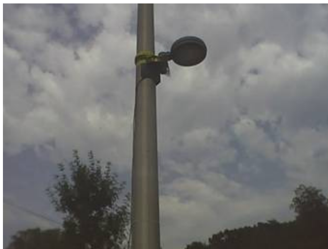
Figure 32. LED overhead luminaire mounted on existing HPS pole.
