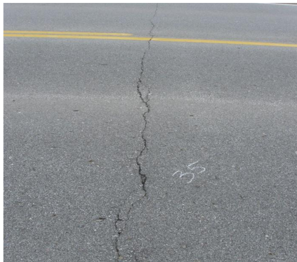
Figure 5.2 Observed Transverse Crack
