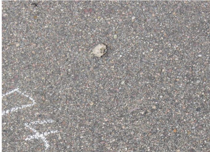
Figure 5.5 Observed Surface Void
