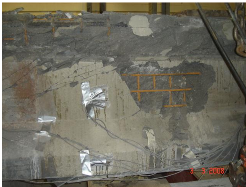
Figure 5.9 Failure of Girder A
