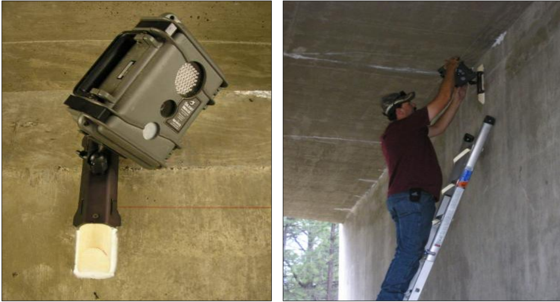
Figure 8. Reconyx™ Camera Mounted on a Wood Strip Glued to the Concrete Surface of Each SR 64 Cataract Canyon Bridge Culvert Cell to Monitor Wildlife Use.
