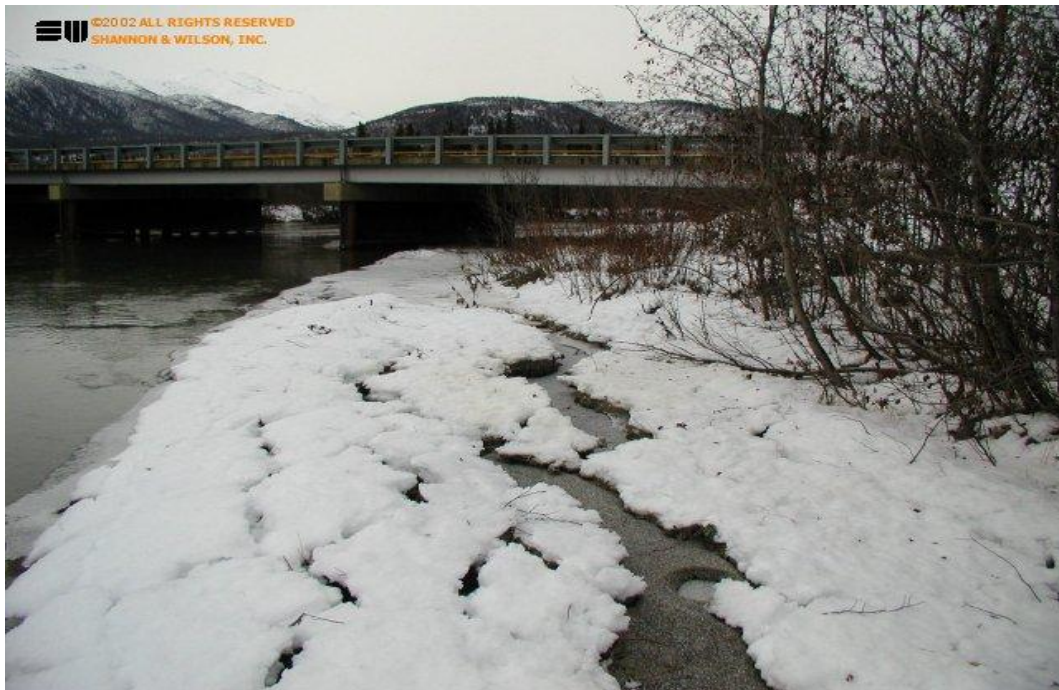
Figure 3.2 Liquefaction-induced lateral spreading in Tok Cutoff Highway embankment (abutment of Slana River Bridge embankment, which is 1 km away from Mabel Creek Bridge)
