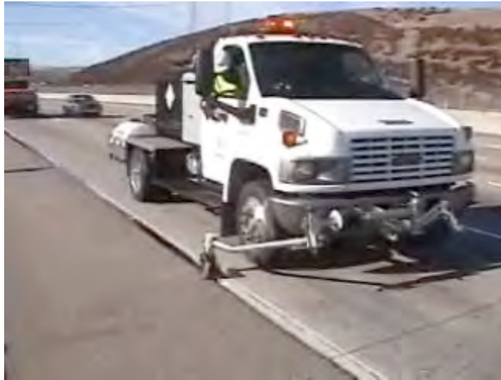
Figure 7. TTLS Moving Closure Sealing Hwy
