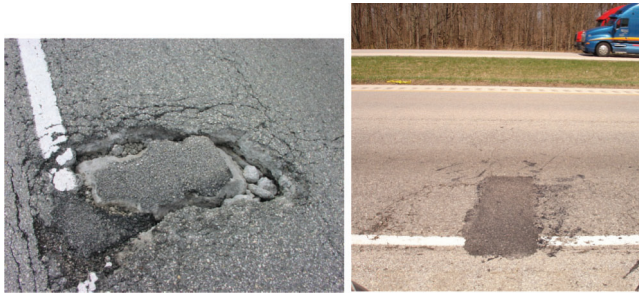
Figure 5.2 Punchout between Sections 5 and 6 (left) and subsequent patching (right).
