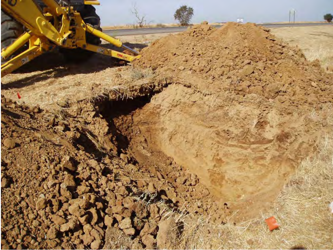
Figure 5. Compacted surface layer of Yuba SR 70 substrate that forms an overhanging ledge (nearest backhoe) and sheets water off the site during rains.
