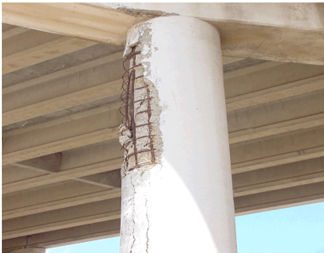
Figure 9-9. Column Deterioration from Chemical Solution Contamination.
