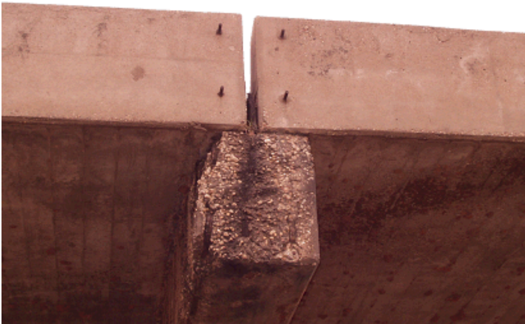
Figure 9-3. Poorly Maintained Joint Allowed Concentrated De-icer Solution to Damage Cap.
