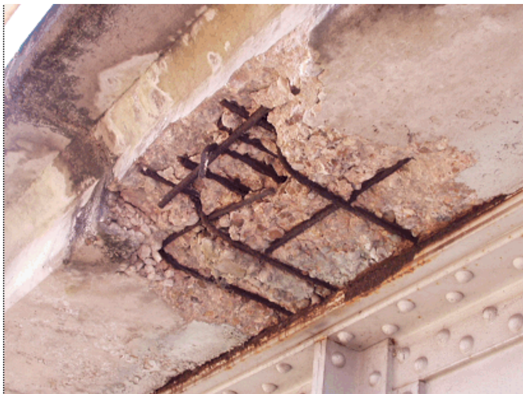
Figure 9-4. Poorly Maintained Joint Allowed De-icer Solution to Damage Overhang to Second Mat of Steel and Top Plate Steel on Beam.
