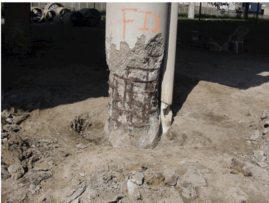
Figure 9-12. Damage Created due to the Salt Storage.
