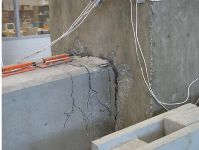
Figure 6.9 Joint Region Following Test Completion - Specimen IB-18-1
