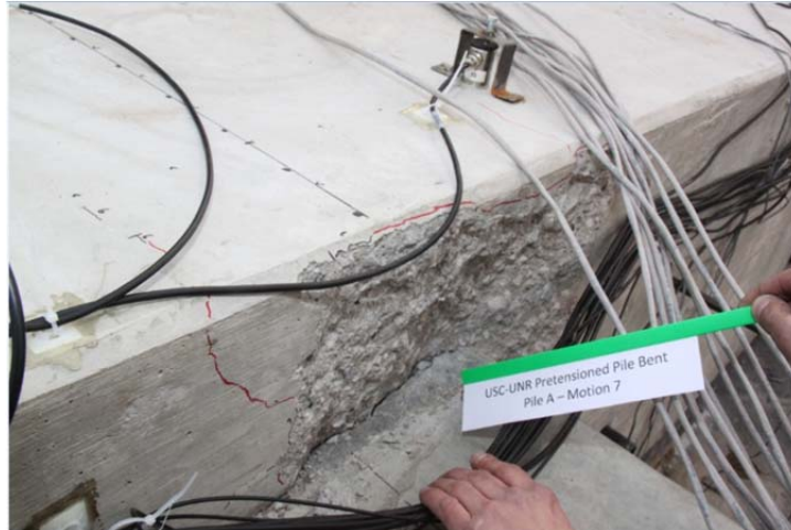
Figure 8.48 Bent Cap Damage - Following 2.0 Josh-T, Pile A
