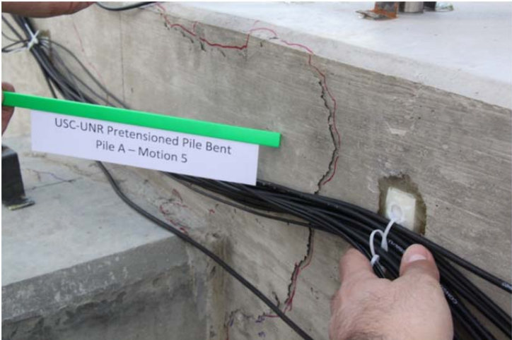
Figure 8.47 Bent Cap Damage - Following 1.0 Josh-T, Pile A
