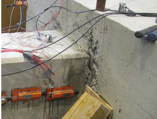
Figure 7.36 Joint Region following Test Completion - Specimen EB-22-1
