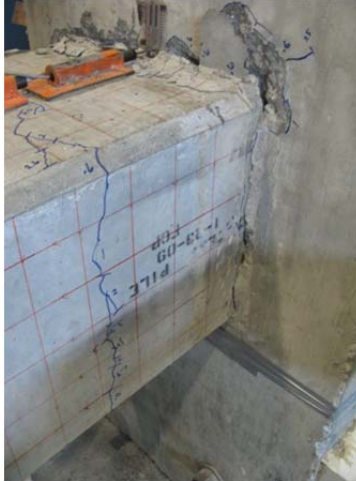
Figure 6.17 Joint Region Following Test Completion - Specimen IB-18-2
