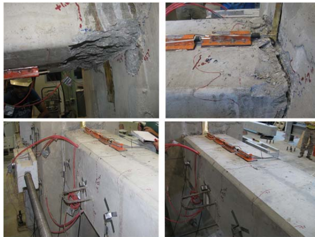
Figure 6.35 Damage Locations - Specimen IB-22-1
