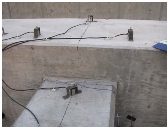
Figure 8.50 Bent Cap Damage - Following 2.0 Josh-T, Pile C
