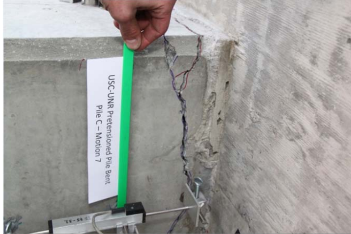
Figure 8.53 Damage to Pile - Following 2.0 Josh-T, Pile C
