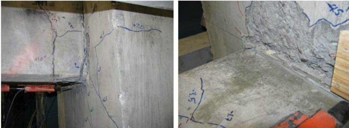
Figure 6.27 Joint Region Following Test Completion - Specimen IB-26-1
