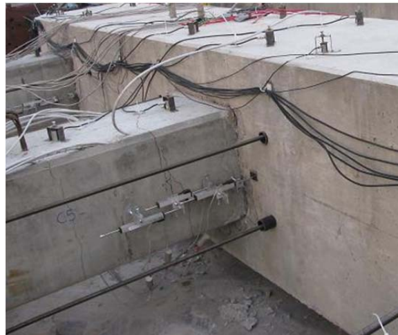
Figure 8.52 Damage to Pile - Following 2.0 Josh-T, Pile B
