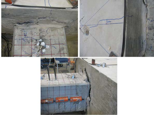
Figure 7.25 Joint Region following Test Completion - Specimen EB-26-1
