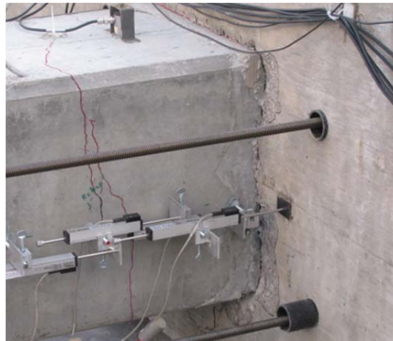
Figure 8.49 Bent Cap Damage - Following 2.0 Josh-T, Pile B
