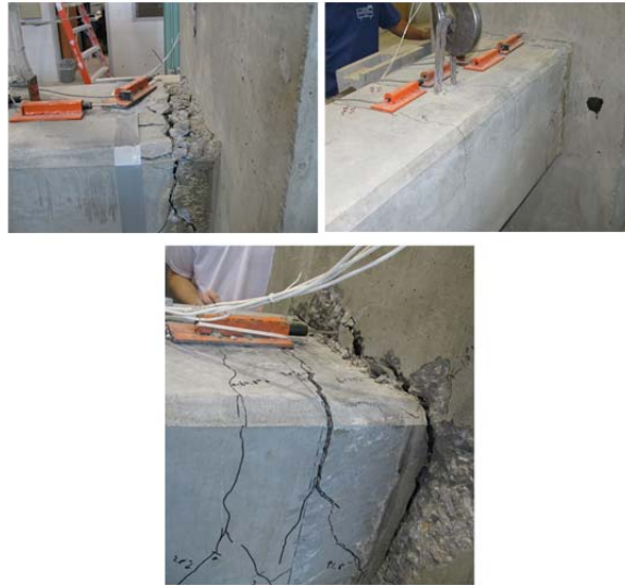
Figure 6.7 Damage Locations - Specimen IB-18-1
