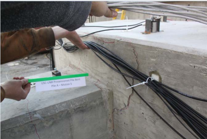
Figure 8.46 Bent Cap Damage - Following 1.0 Josh-T, Pile A
