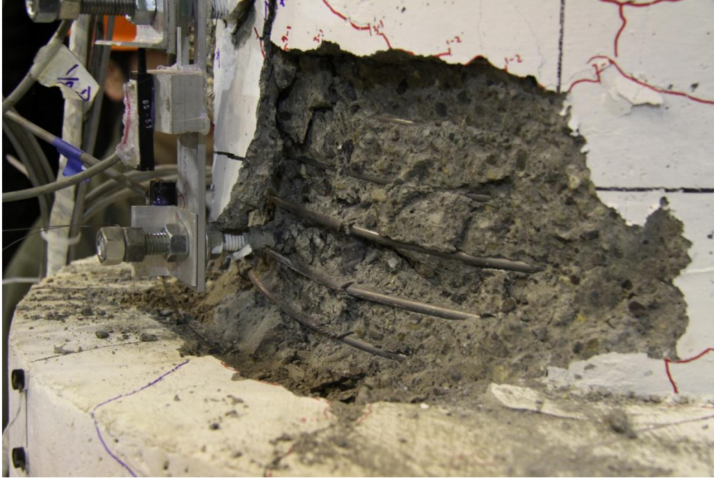
Figure C-0-4. DS-1 – First noticeable bar buckling in the column in Cycle 9-3 (6.90/-6.81 percent drift)
