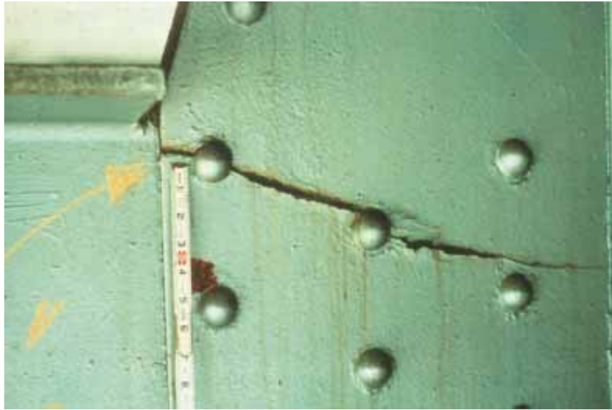
Figure 4.1: Fatigue crack at coped top flange of riveted connection, after United States Department of Transportation: Federal Highway Administration (2006)
