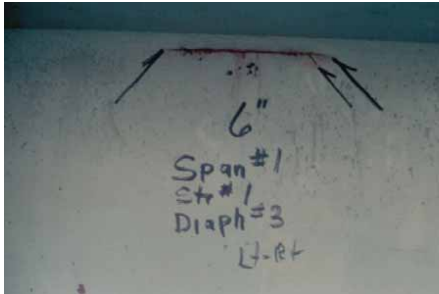
Figure 4.2: Fatigue crack marked as per the BIRM, after United States Department of Transportation: Federal Highway Administration (2006)
