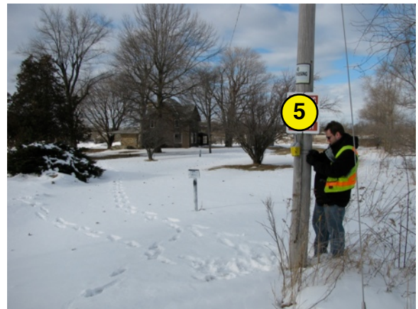
Figure 2.5 - Node 5 as relay point on telephone pole
