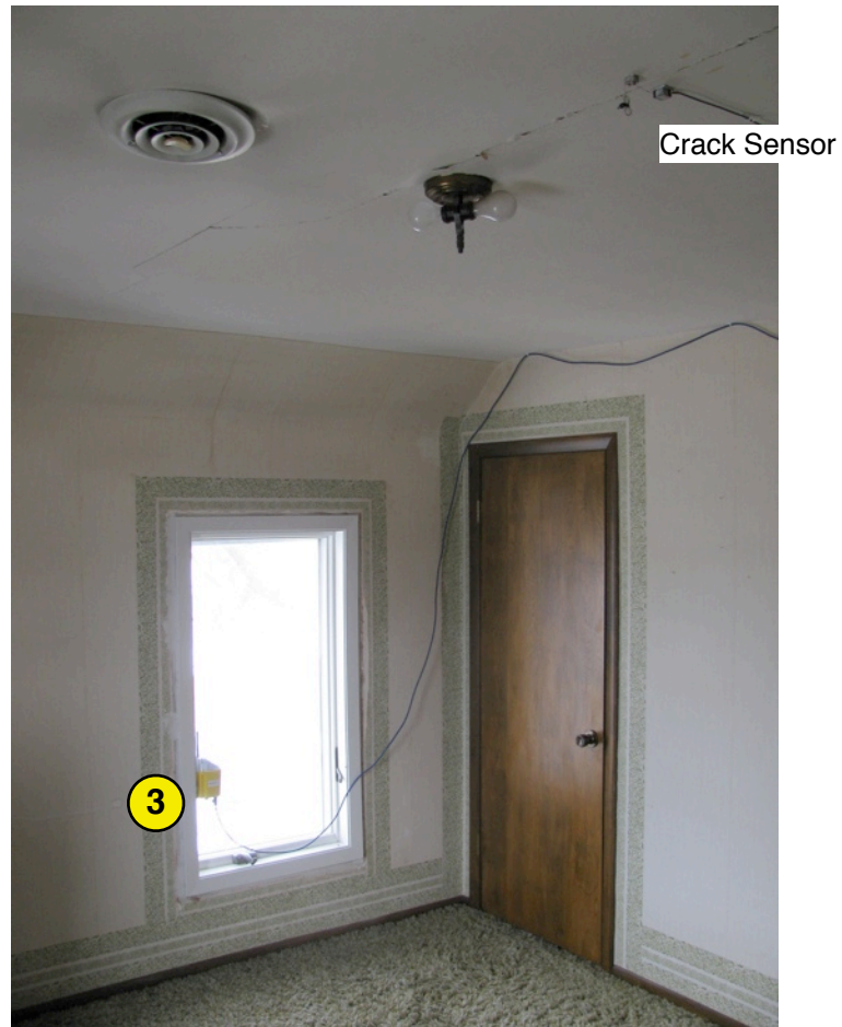
Figure 2.10 - Interior view of Node 3 in upstairs bedroom. Crack sensor connected to eKo Mote.
