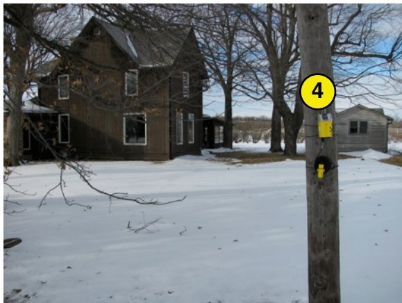
Figure 2.4 - Node 4 as relay point on telephone pole
