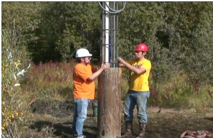
Figure 2.10: Installing a reinforcing steel cage with sensors into a test pile (photo by INE staff).
