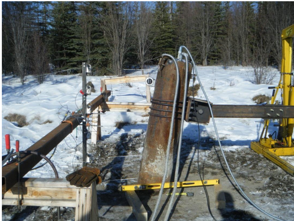
Figure 2.30: At 207 kips, final loading of the south pile.
