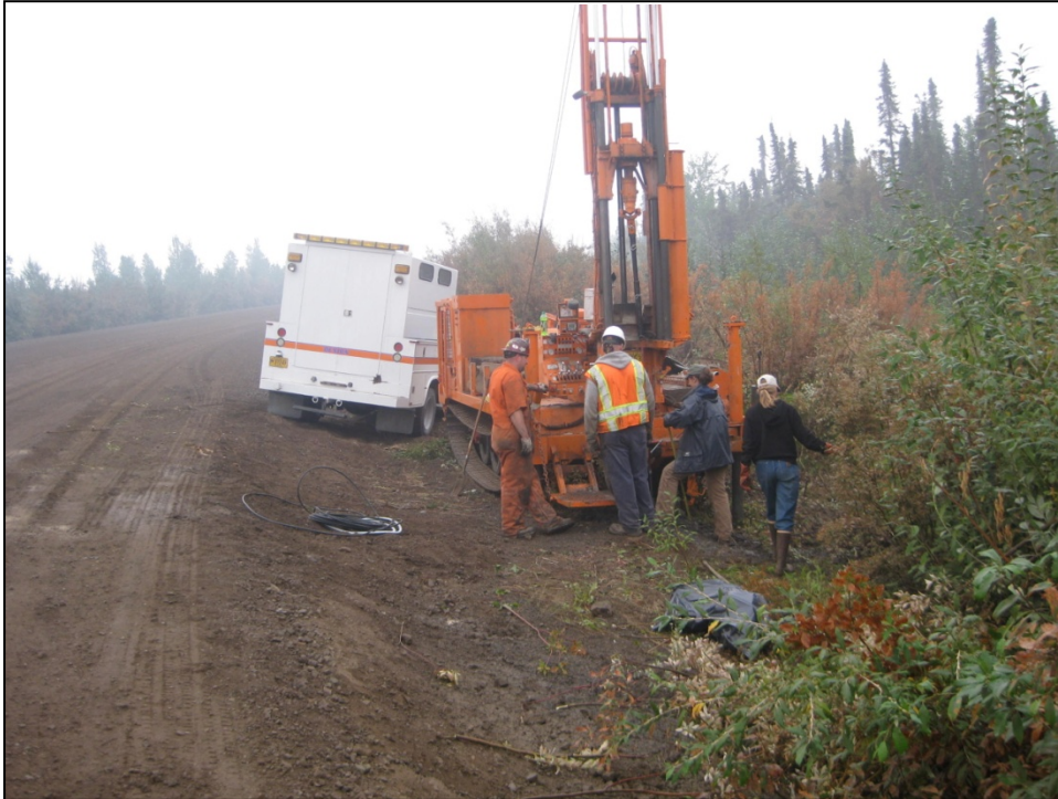
Figure 3.10. Location of TH09-1404, at the toe of the embankment. Note the cables from TH09-1403 emerging from the side slope.
