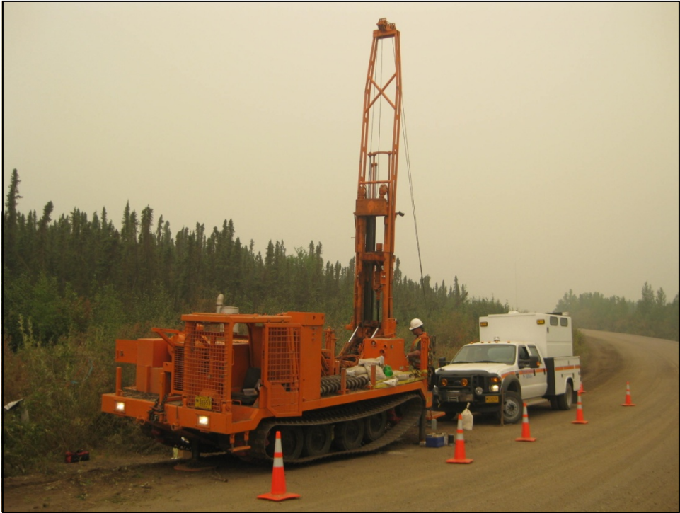
Figure 3.6. Location of TH09-1403 on the Dalton Highway shoulder. View to the northwest.
