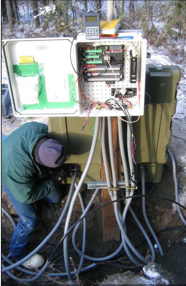
Figure 2.12. Thermistor cables and Liquid Tight conduit routing into the ADAS system.
