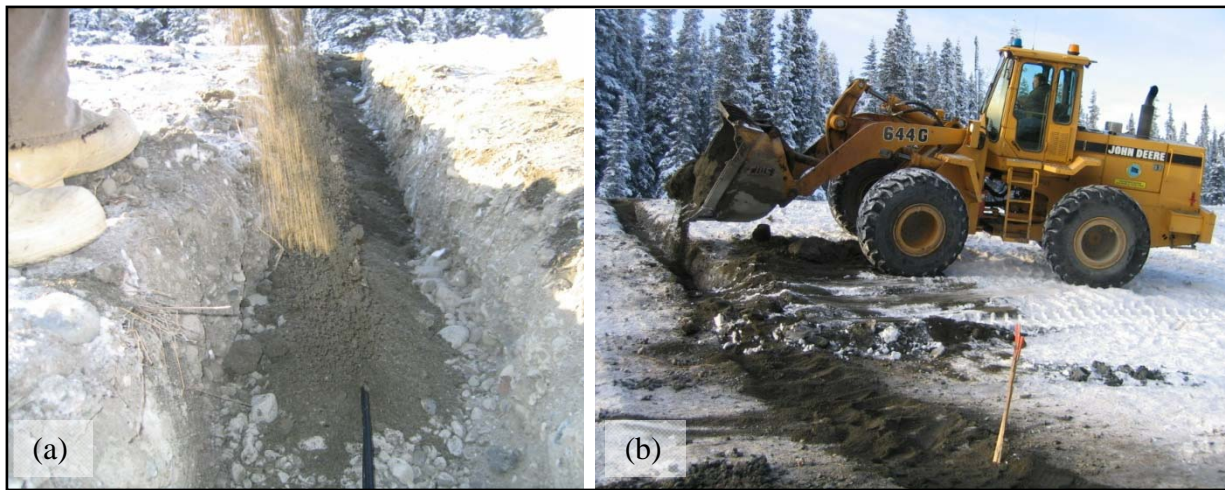
Figure 2.11. Backfilling the trench: (a) anchoring the cables using buckets and shovelfuls of sand; (b) M&O making short work of the backfilling with a loader.
