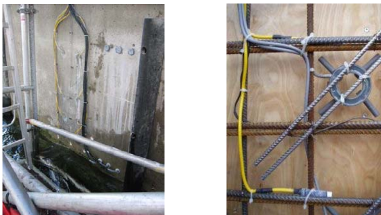
Fig. 18.1 CorroWatch and ERE 20 attached to the reinforcement
