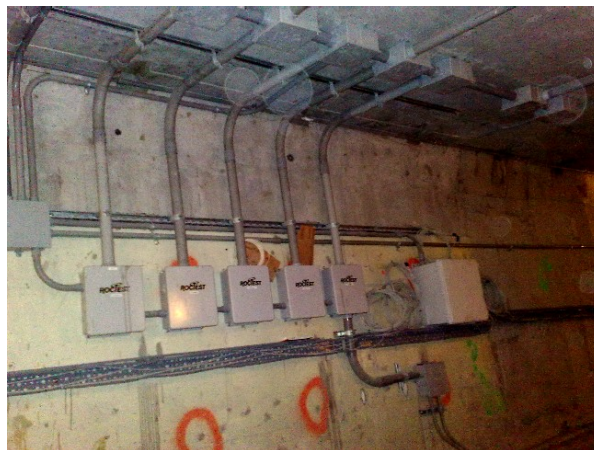
Junction boxes inside the main span of the South bound
