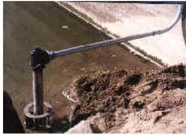
Fig. 19.2 MSC scour monitoring system
