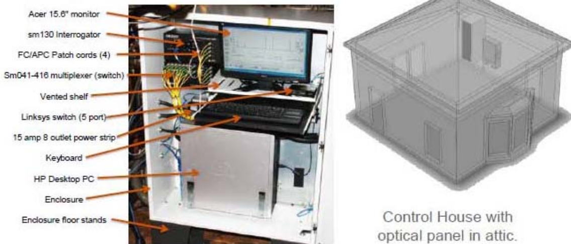
Fig. 21.14 Control house and system
