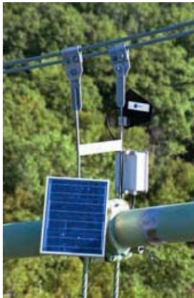
Fig. 17.3 Wireless Sensors attached to cable (Waldo Hancock Bridge, Verona, Maine)
