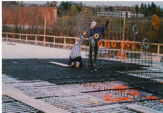
Fig. 21.24 Installation of the instrumented sections of bridge deck reinforcement in the Joffre Bridge
