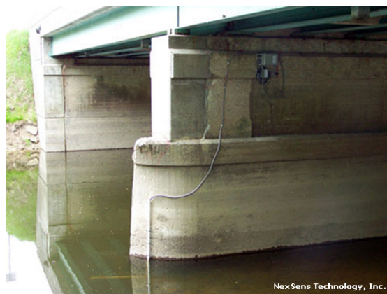
Fig. 19.1 Bridge scour monitoring site
