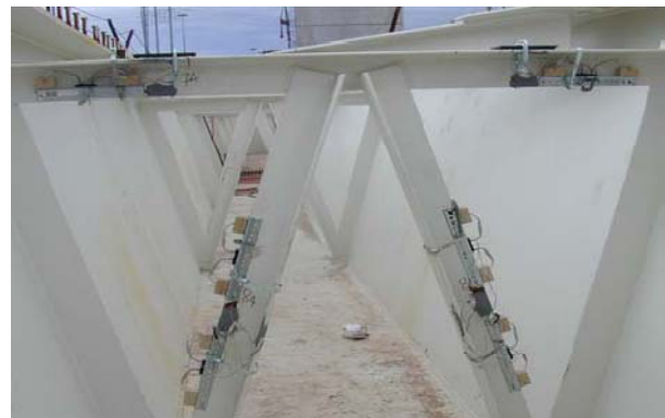
Fig. 15.3 MicroWIS units mounted on K-frame
