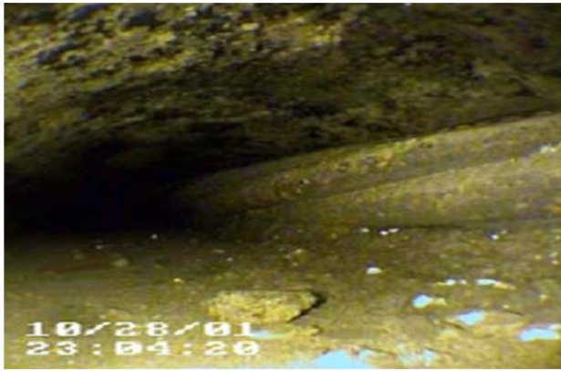
Partially grouted duct
