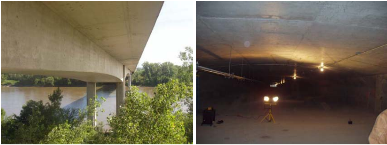
Figure A.7: An example of major segmental post-tensioned bridge inspected by P.I.
