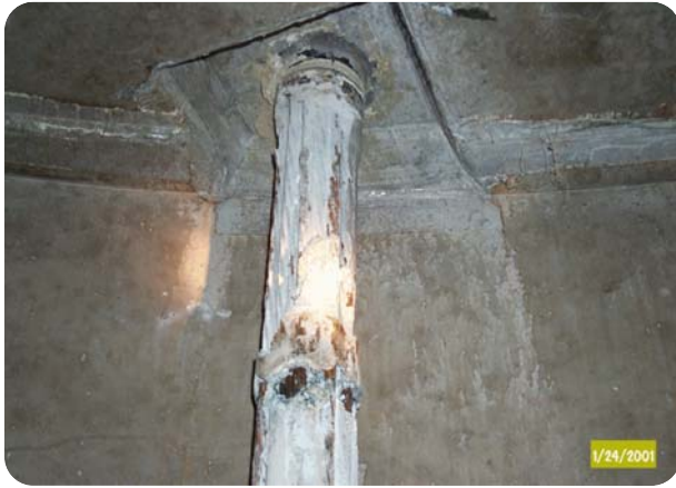
(a): Corrosion activity in the voided area
