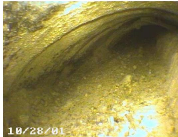
Partially grouted duct but no strand exposure
