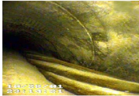
Partially grouted duct with partially exposed strands
