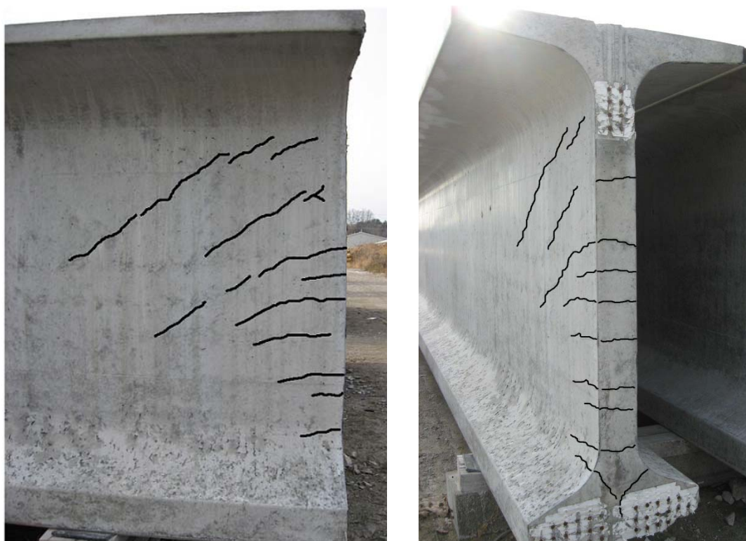
Figure 1 – Typical cracking pattern of the deep wide flanged girders.
