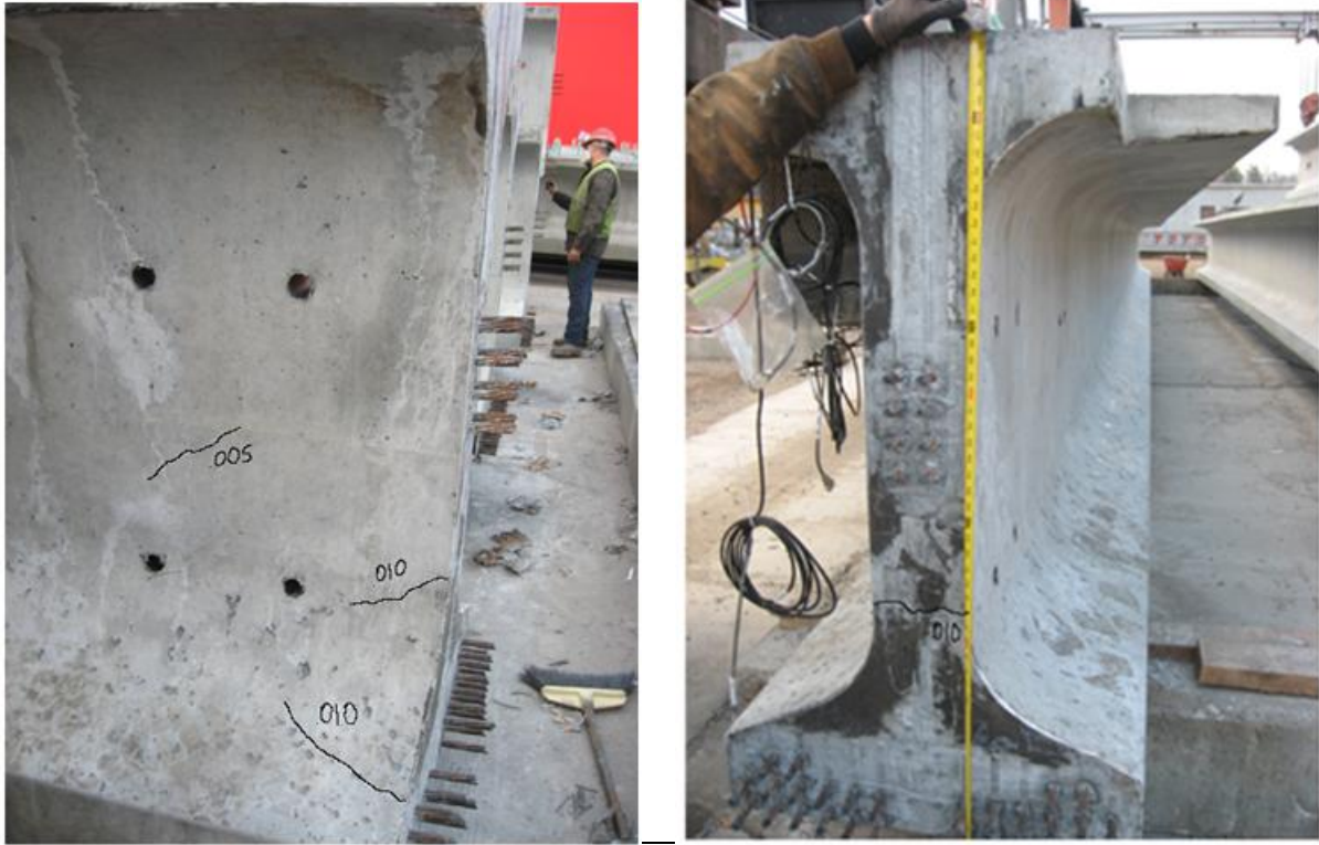
Figure 37 – Initial crack locations and widths in the monitored girder.
