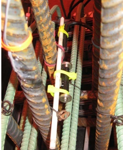
Figure 33 – 2in vibrating wire gage positioned in concrete through nonstructural attachments to rebar.
