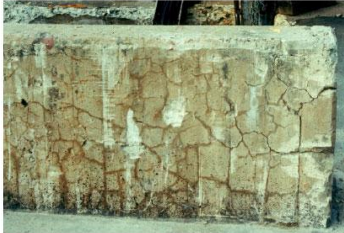
Figure 1-2: ASR crack manifestation (Folliard et al. 2006)
