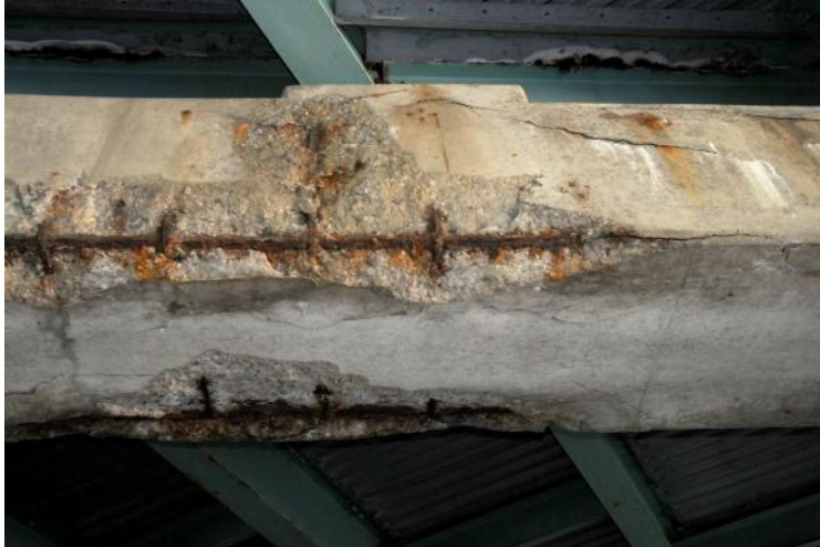
Figure 3-7: Corrosion of steel reinforcing bars in concrete (Courtesy of Matco Services, Inc.).
