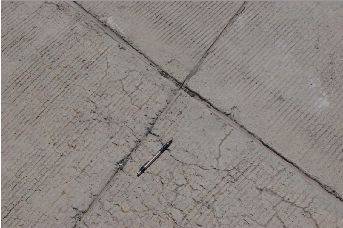
Figure 2. I-84 Concrete Exhibiting Cracking Caused by ASR
