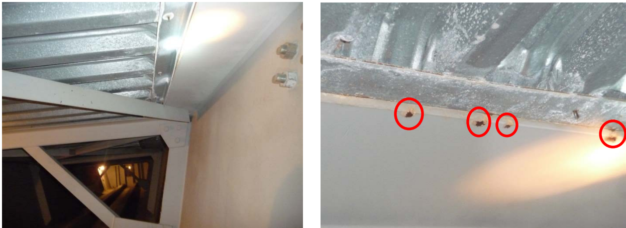
Figure 3-9: Internal investigation for corrosion shows detected corrosion spots
