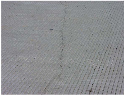
Figure 1-3: Deck with transverse linear cracks
