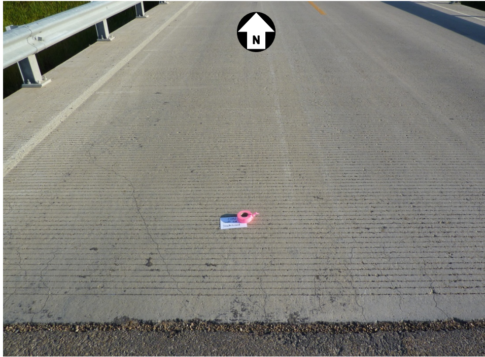
Figure 13: Cracking on the southwest end of the Conventional deck in 2009.
