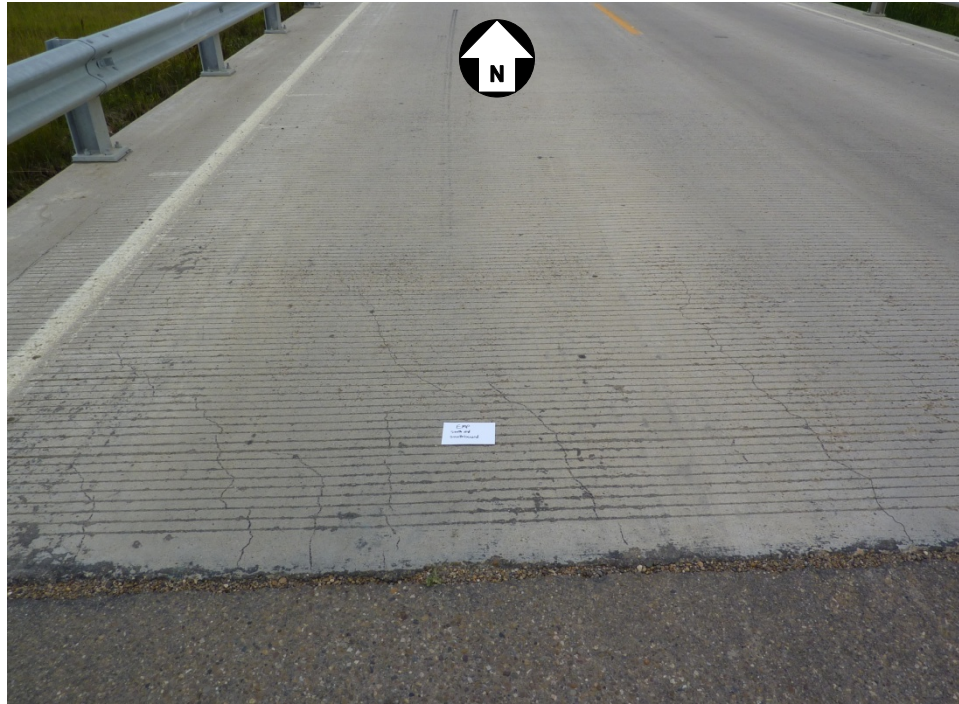
Figure 14: Cracking on the southwest end of the Empirical deck in 2009.
