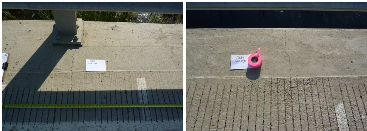
Figure 15: Cantilever edge cracking, eastern edge, HPC–left, Conventional–right, in 2009.
