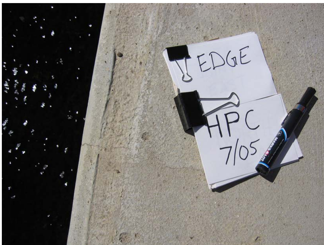
Figure H -30: Edge Cracking on West Side – HPC Deck
