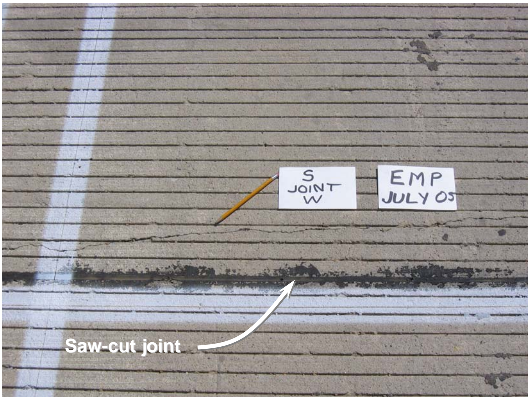
Figure H -13: Full-Depth Transverse Crack at Southern-Most Interior Bent – Empirical Deck
