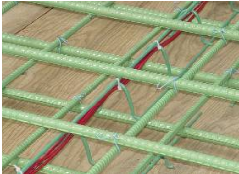
Figure 33: Example of Cable Run
