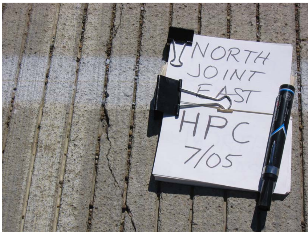
Figure H -26: Full-Depth Transverse Crack at Northern-Most Interior Bent – East HPC Deck
