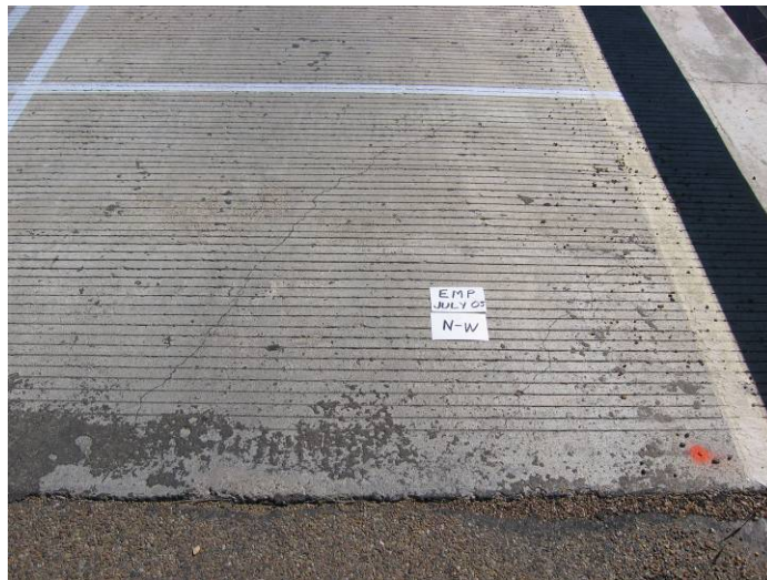
Figure 109: Top-Surface Cracking at West Side of North Abutment – Empirical Deck
