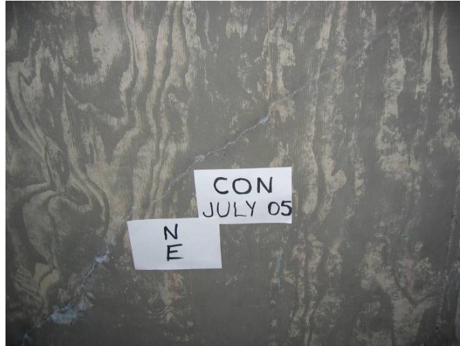
Figure 111: Full-Depth Crack at Northeast Corner (shown from underside) – Conventional Deck
