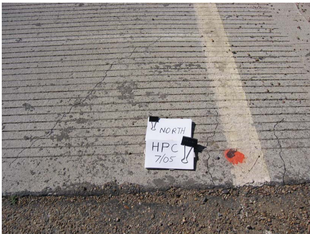
Figure H -28: Top-Surface Cracking at West Side of North Abutment – HPC Deck
