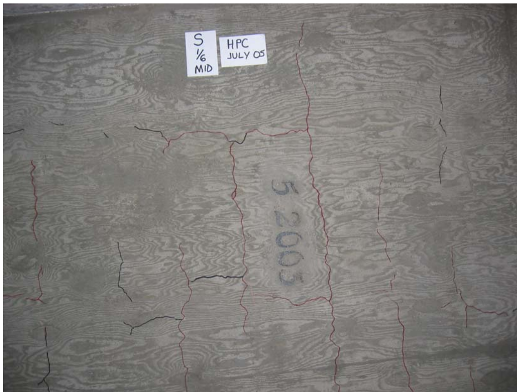
Figure H -31: Hairline Cracking near South Abutment (shown from underside) – HPC Deck
