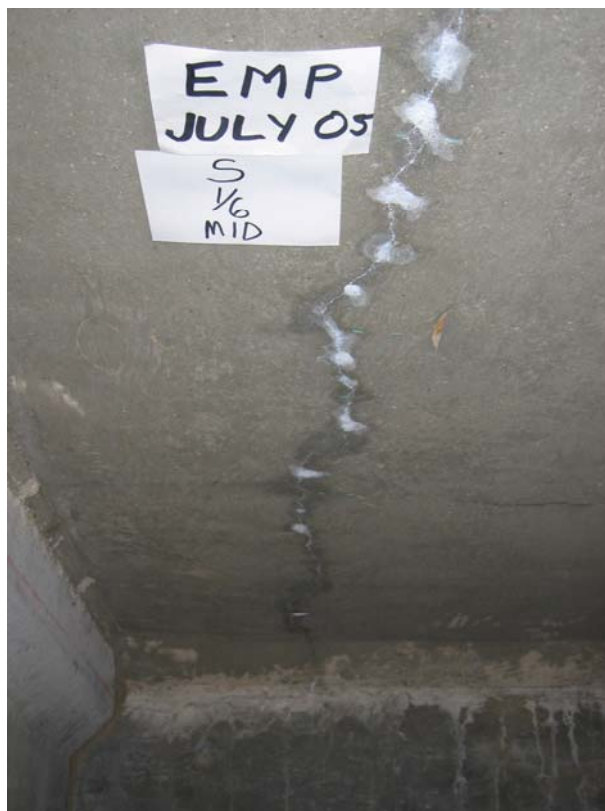
Figure H -20: Full-Depth Crack near Center of South End (shown from underside) – Empirical Deck
