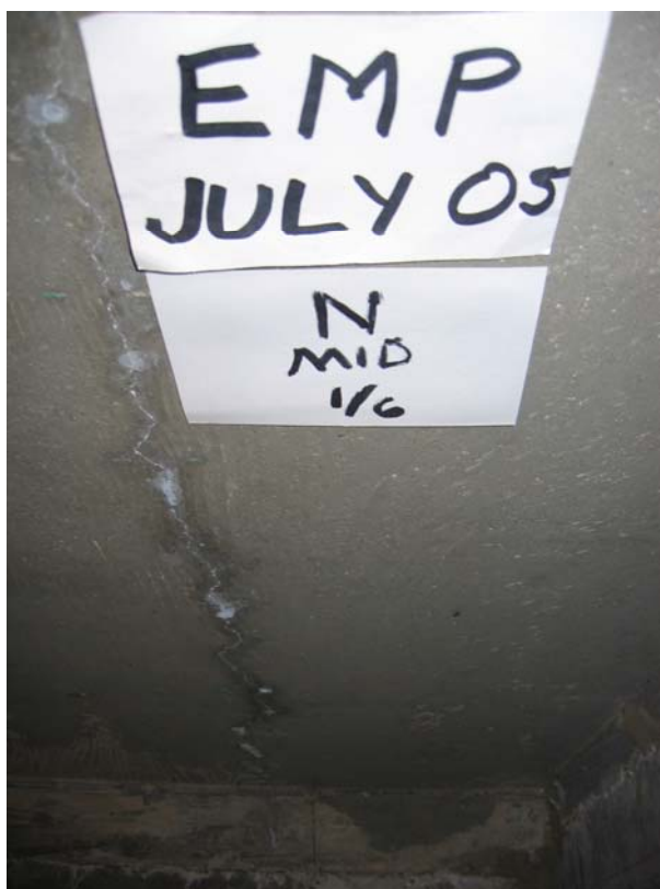
Figure H -17: Full-Depth Crack near Center of North End (shown from underside) – Empirical Deck
