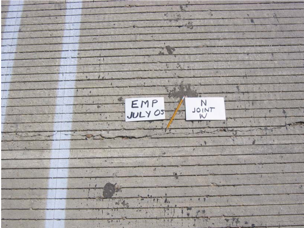
Figure H -12: Full-Depth Transverse Crack at Northern-Most Interior Bent – Empirical Deck
