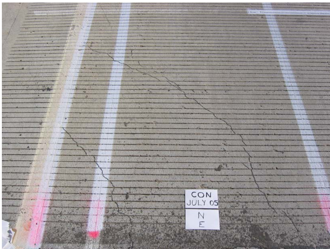
Figure H -5: Top-Surface Cracking at East Side of North Abutment – Conventional Deck
