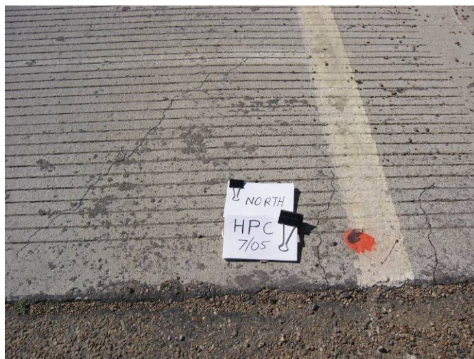
Figure 110: Top-Surface Cracking at West Side of North Abutment – HPC Deck
