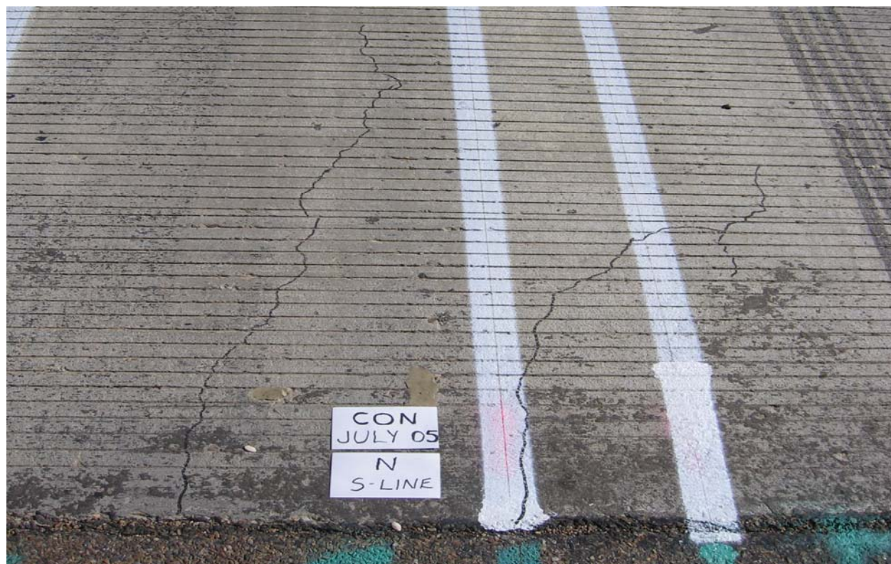
Figure H -4: Top-Surface Cracking at West Side of North Abutment – Conventional Deck
