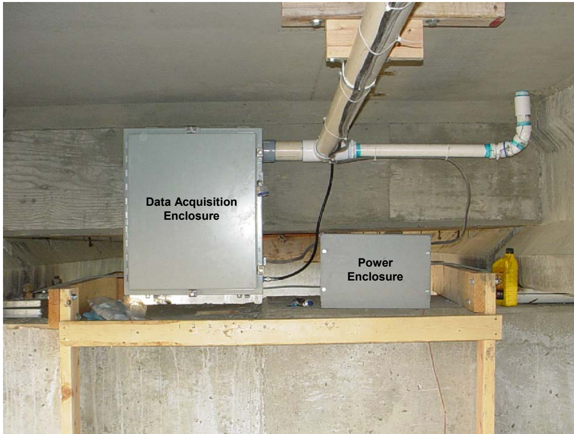
Figure 34: Data Acquisition and Power Enclosure Arrangement under the Bridge Decks
