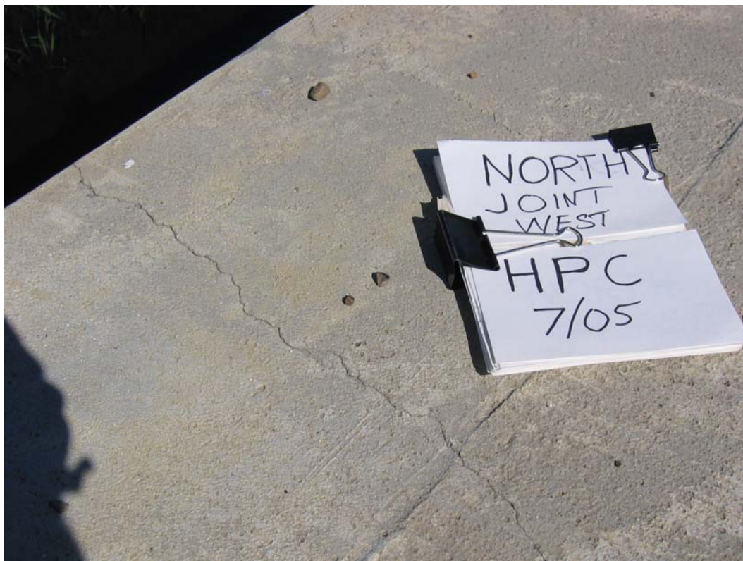
Figure H -25: Full-Depth Transverse Crack at Northern-Most Interior Bent – West HPC Deck
