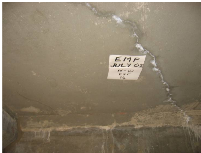
Figure 112: Full-Depth Crack at Northwest Corner (shown from underside) – Empirical Deck
