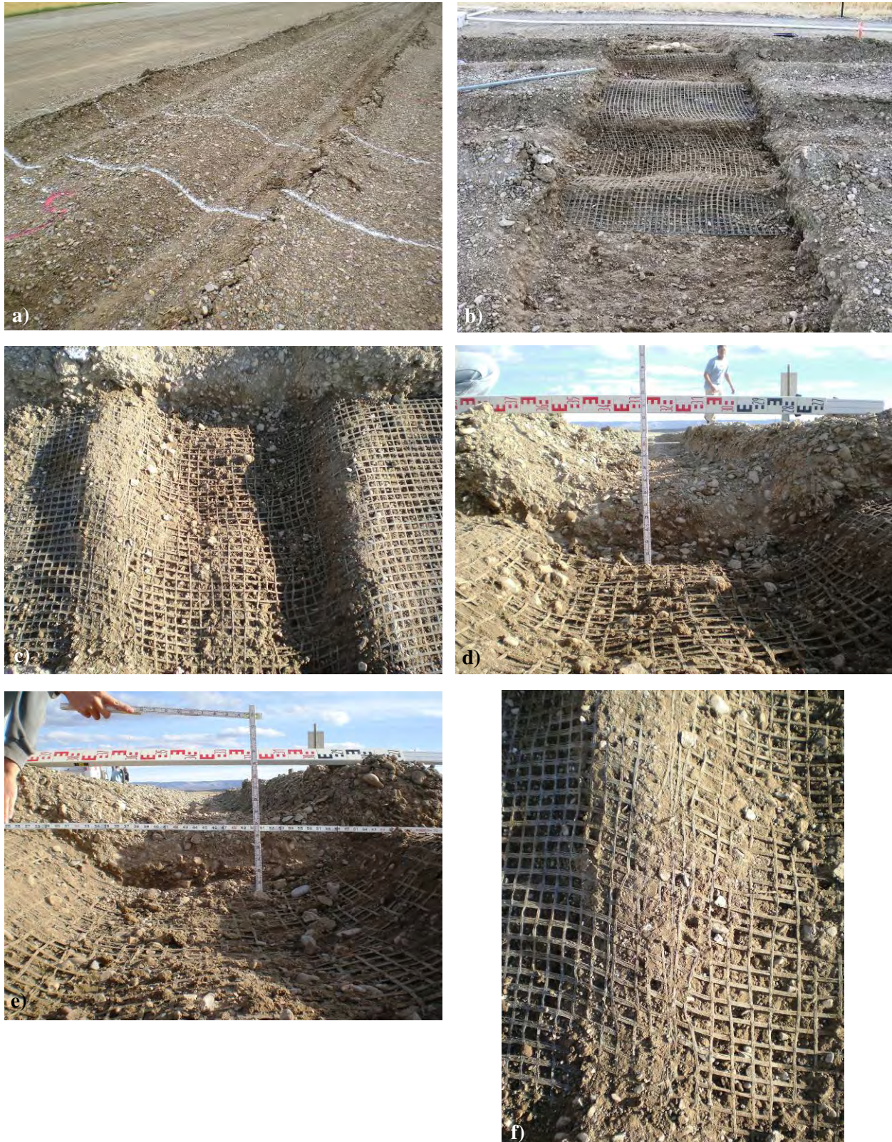
Figure C-28. Photos of the forensic excavations of the WoG-8 test section: a) excavation area, b) looking west, c) rut bowl, d) base rut profile, e) subgrade rut profile and f) close-up of rut.
