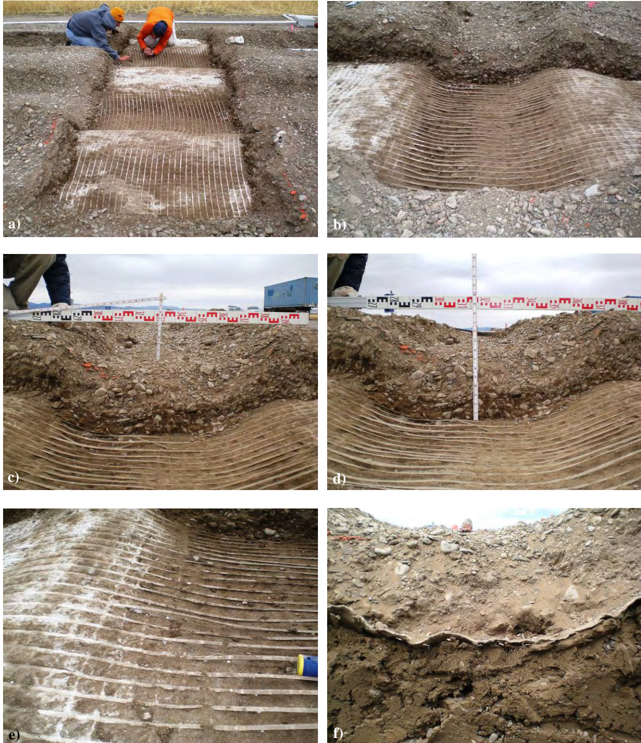
Figure C-17. Photos of the forensic excavations of the CoG-4 test section: a) looking west, b) rut bowl, c) base rut profile, d) subgrade rut profile, e) close-up of rut and f) layering of base and subgrade.
