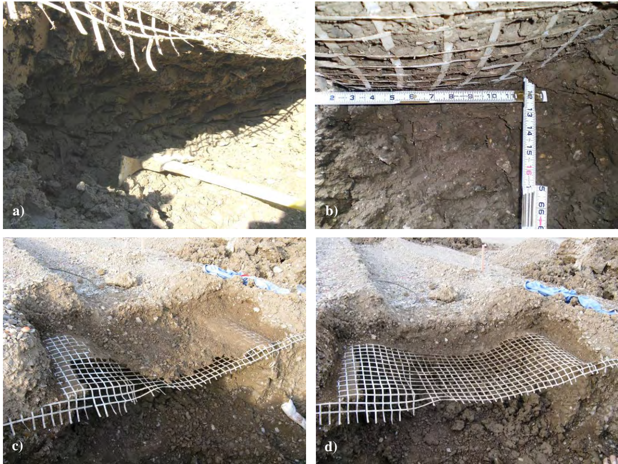
Figure 36. Pictorial overview of the reverse excavation method: a) excavating underneath the geosynthetic, b) subgrade fully removed and geosynthetic exposed, c) removal of the base from the top and d) fully exposed geosynthetic.
