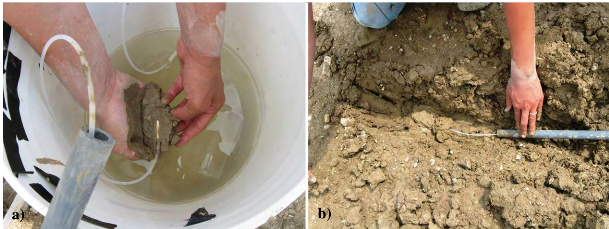
Figure 10. Installation of pore water pressure sensors: a) encapsulating porous stone with saturated subgrade, b) burying in subgrade.
