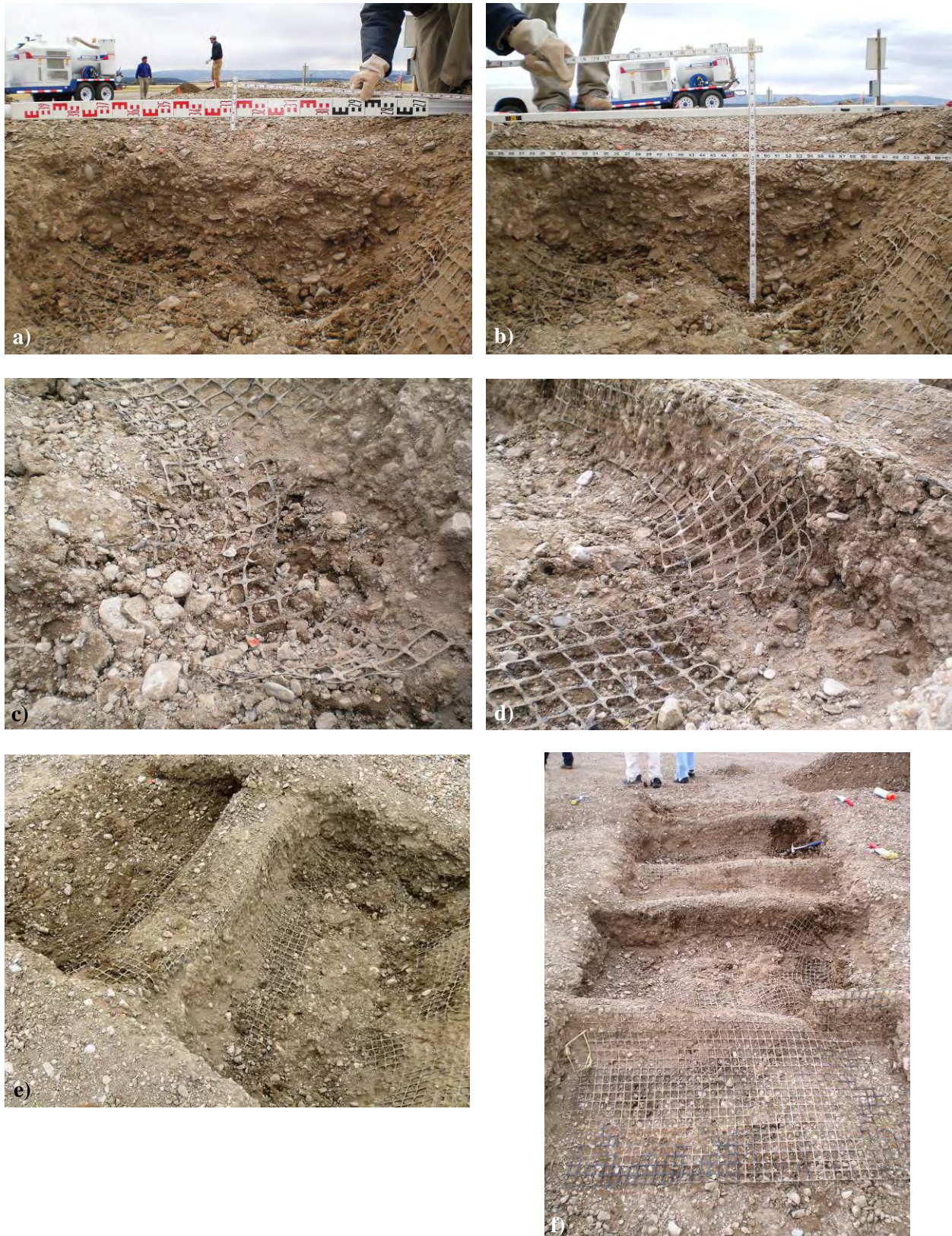
Figure C-19. Photos of the forensic excavations of the IFG-5 test section: a) base rut profile, b) subgrade rut profile, c) close-up of rut, d) close-up of damage, e) rut bowl and f) looking east.
