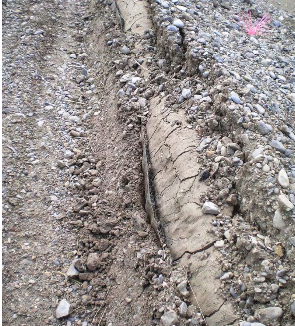
Figure 42. Pullout failure of the WoT-9 geotextile.
