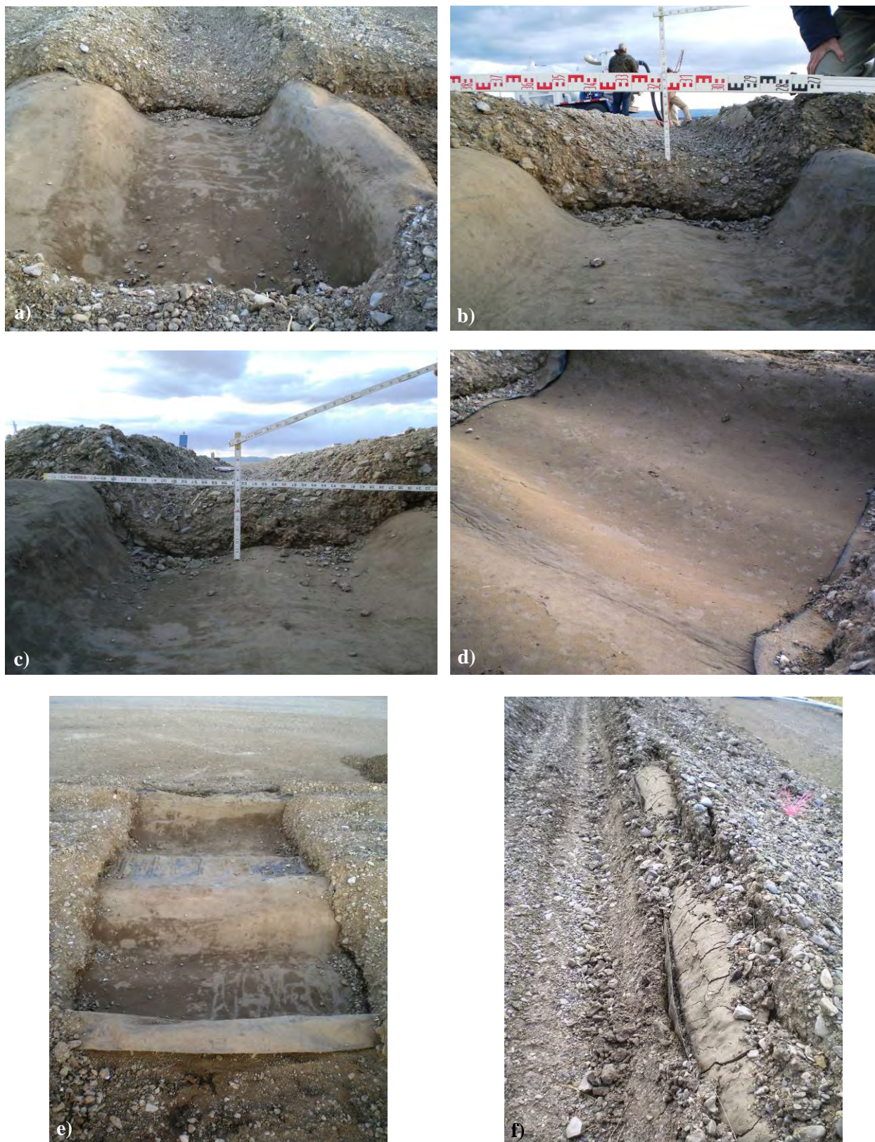
Figure C-31. Photos of the forensic excavations of the WoT-9 test section: a) rut bowl, b) base rut profile, c) subgrade rut profile, d) subgrade surface, e) looking east and f) pullout failure.
