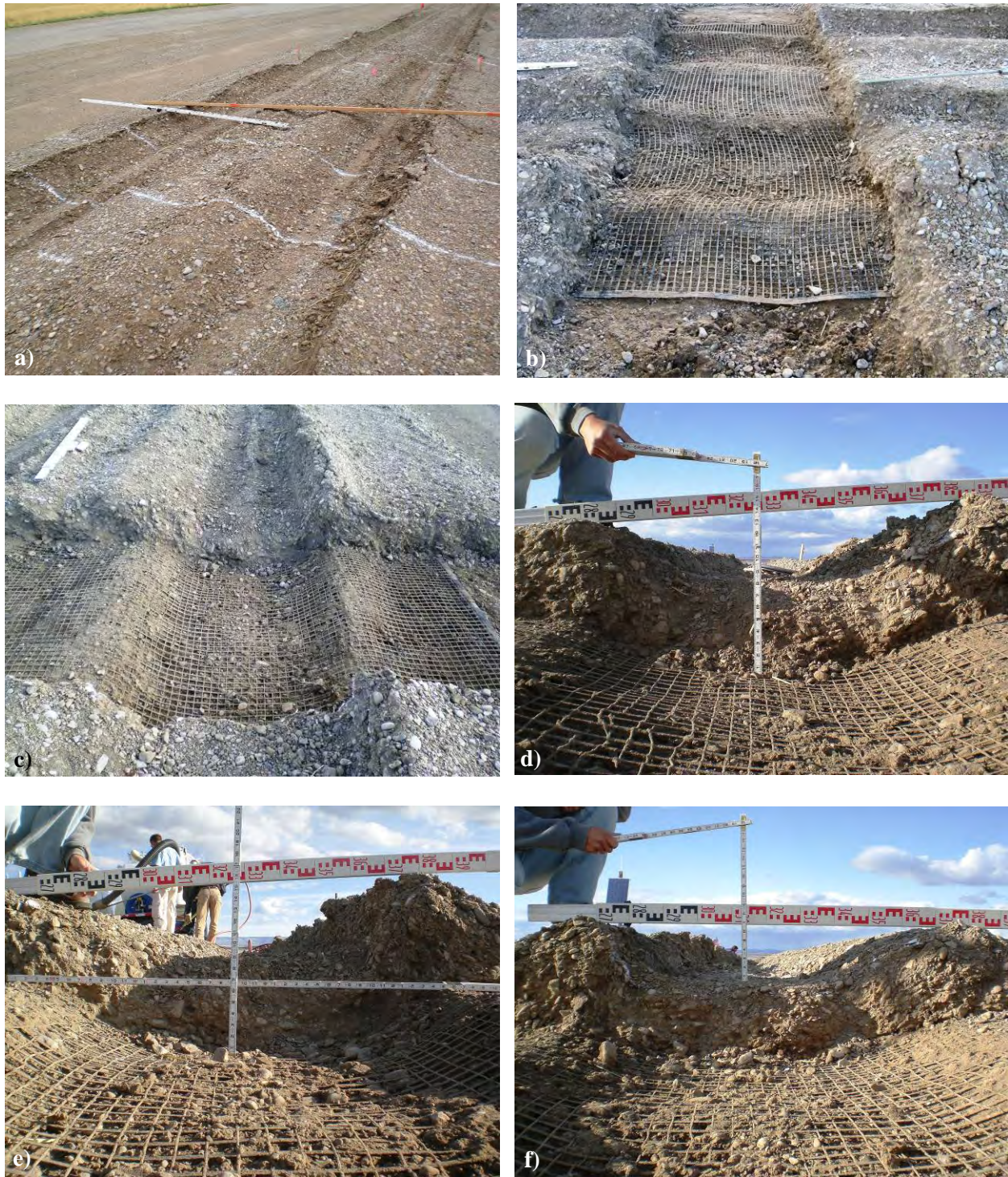
Figure C-25. Photos of the forensic excavations of the WoG-7 test section: a) excavation area, b) looking west, c) rut bowl, d) subgrade rut profile, e) subgrade rut profile and f) base rut profile.
