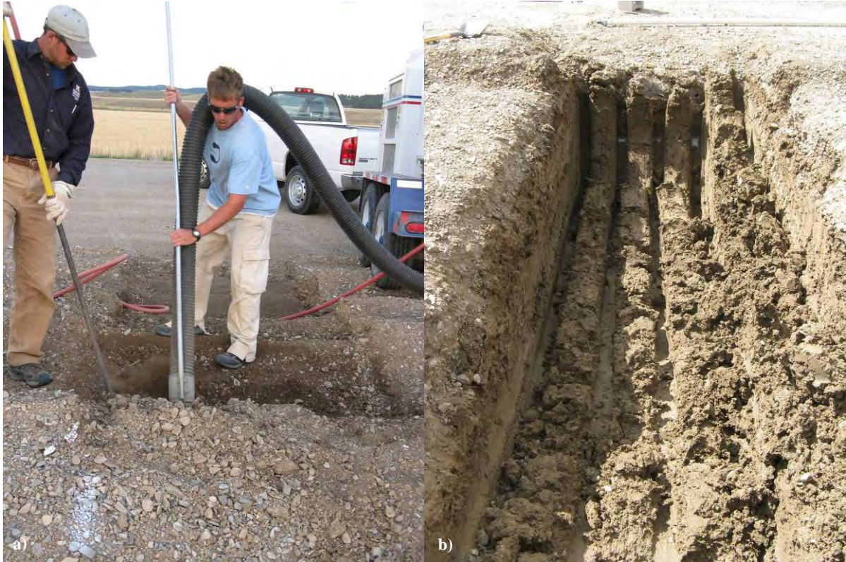
Figure 34. Forensic investigations: a) air and vacuum removal of base course, b) excavation of subgrade.
