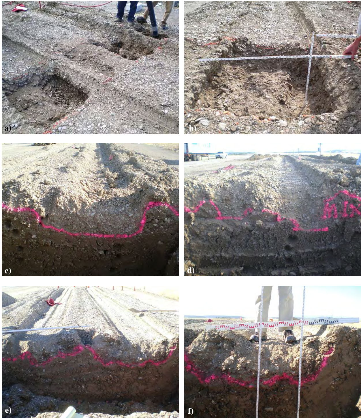
Figure C-5. Photos of the forensic excavations of the Control sections: a) and b) excavation of Control 1, c) and d) rut profile of Control 1, e) and f) rut profile of Control 2.
