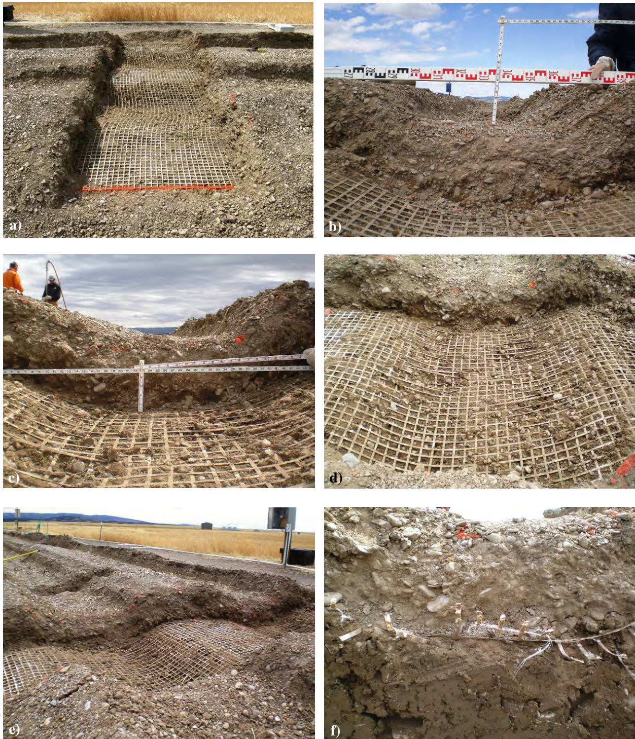
Figure C-22. Photos of the forensic excavations of the WeG-6 test section: a) looking west, b) base rut profile, c) subgrade rut profile, d) rut bowl, e) view from the side and f) layering of base and subgrade.
