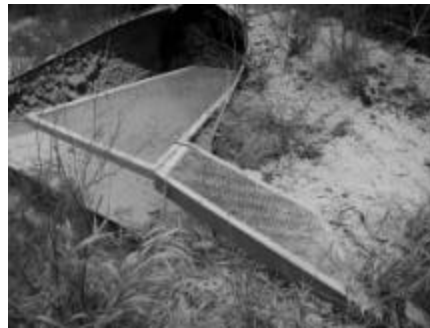
Figure 15. Entrance ramp at Carleton Creek Experimental positioned to side of shelving and culvert.
