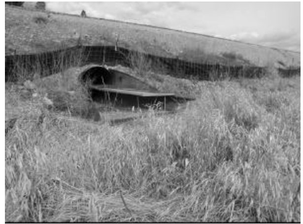
East entrance heavily vegetated
