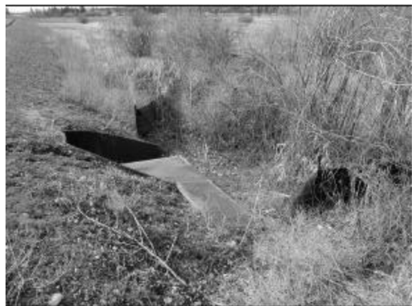
East entrance heavily vegetated
