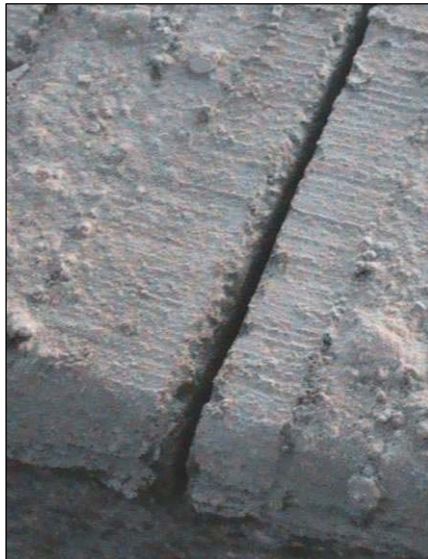
Figure 16. Example of saw cut along transverse tining where the left edge of the joint face appears to be lightly raveled while the right edge is more cleanly cut.
