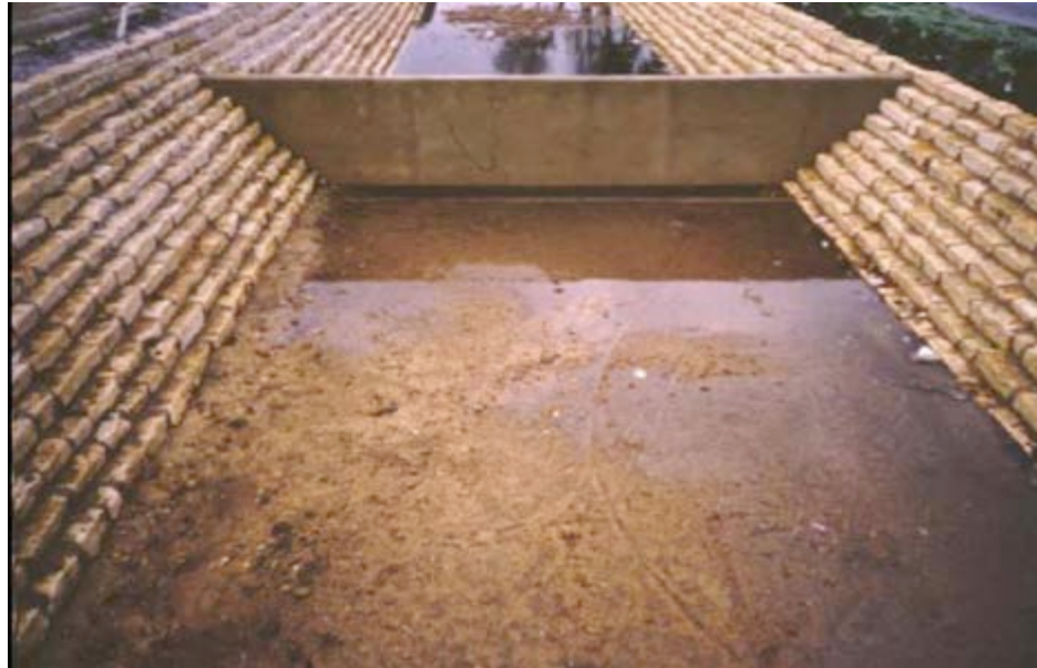
Figure 9. Newly constructed bioretention area (Georgia Stormwater Manual).
