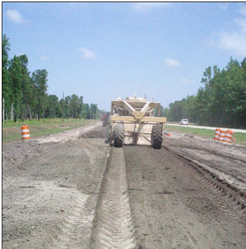
Figure 3-29: The soil stabilizer mixing the cement into the top 8 inches of subgrade soil
