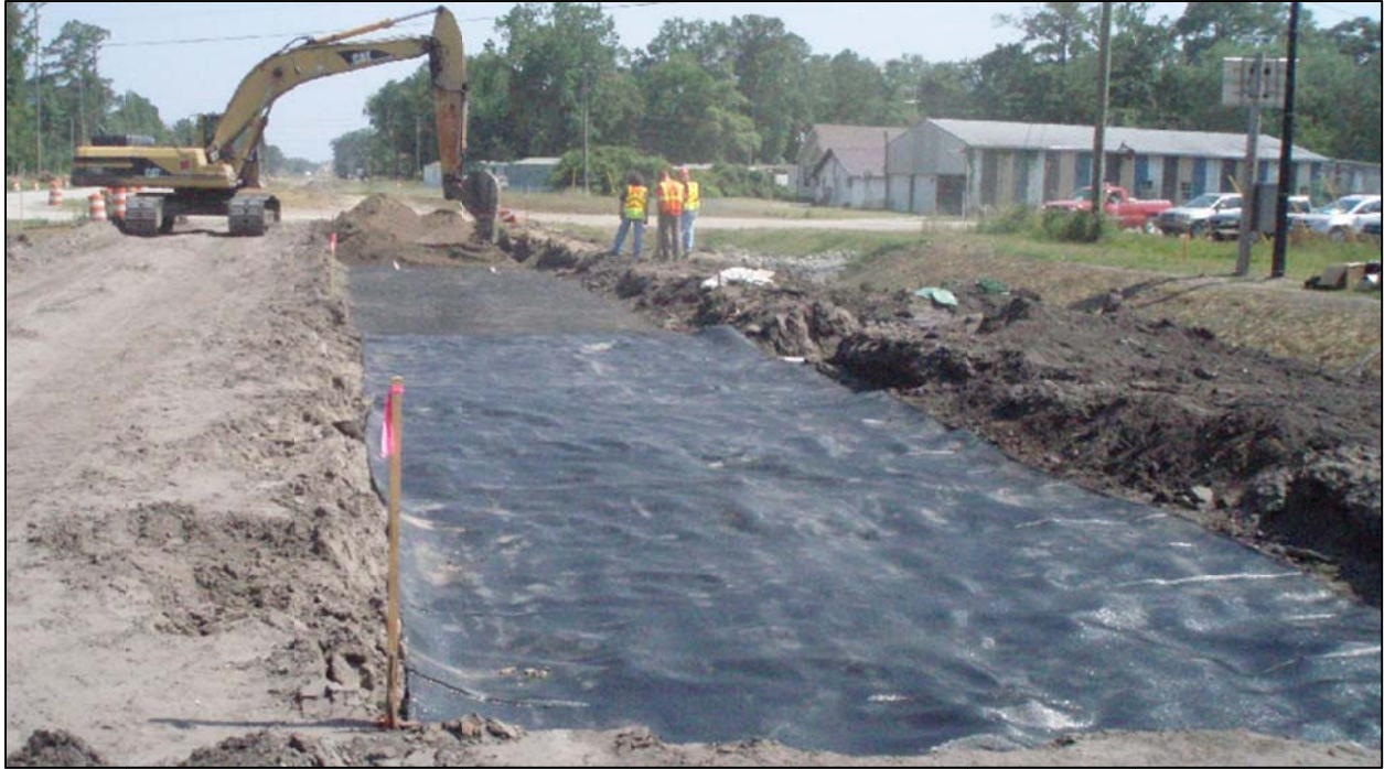
Figure 3-26: The geogrid installed in Test Section 2 and the geotextile installed in Test Section 3
