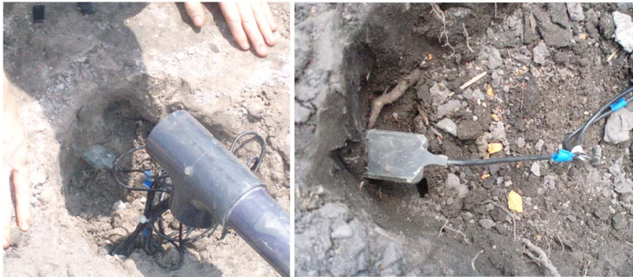
Figure 3-24: Moisture sensors installed (left) in Test Section 1 and (right) in Test Section 2
