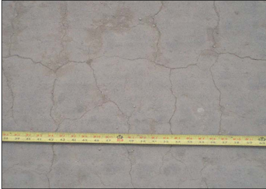
Figure 5-80: Image of the OWP in Test Section 3 after 1000 passes. Note the alligator cracking which was prevalent in Test Sections 2 and 3.
