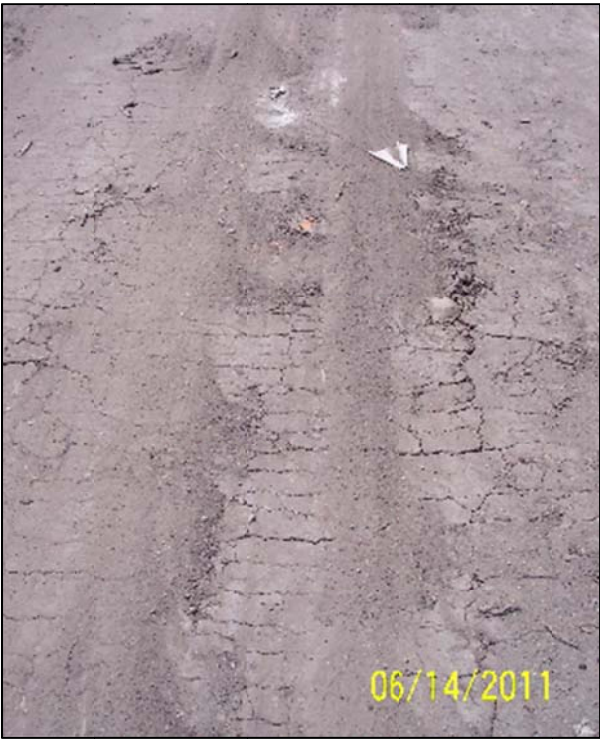
Figure 5-81: Cracks developing along the IWP in Test Section 4 after 10 truck passes
