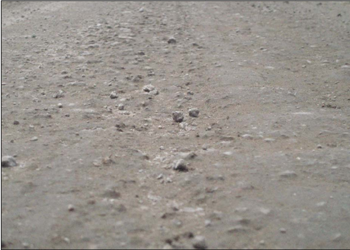
Figure 5-89: An image taken close to the ground surface of the OWP in Test Section 2
