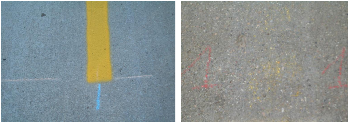
Figure 6.1 Concrete pavement condition before (left) and after (right) 12 mils water-based paint has been removed by water blasting
