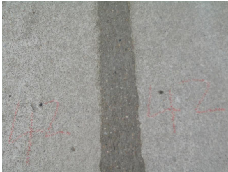
Figure 6.20 Condition of concrete pavement after heat torch applied on tape
