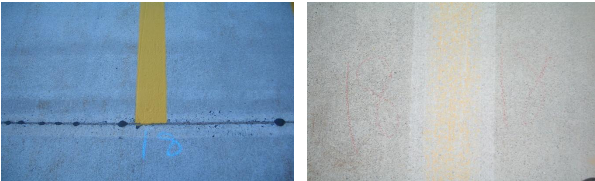
Figure 6.12 Concrete pavement condition before (left) and after (right) paint has been removed with scarifier
