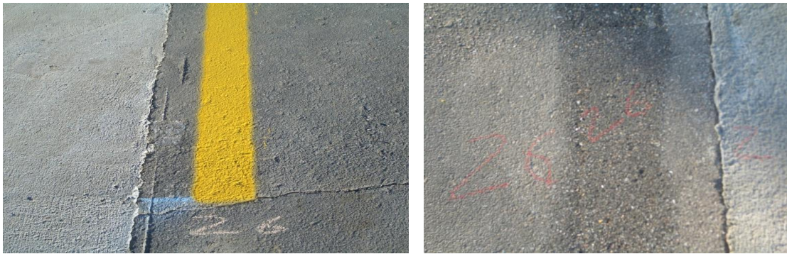
Figure 6.3 Asphalt pavement condition before (left) and after (right) 10 mils water-based paint has been removed by water blasting
