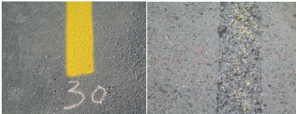
Figure 6.13 Asphalt pavement condition before (left) and after (right) paint has been removed with scarifier
