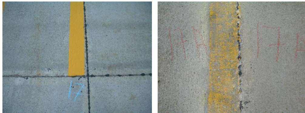
Figure 6.8 Concrete pavement condition before (left) and after (right) 12 mils oil-based paint has been removed by dry ice blasting
