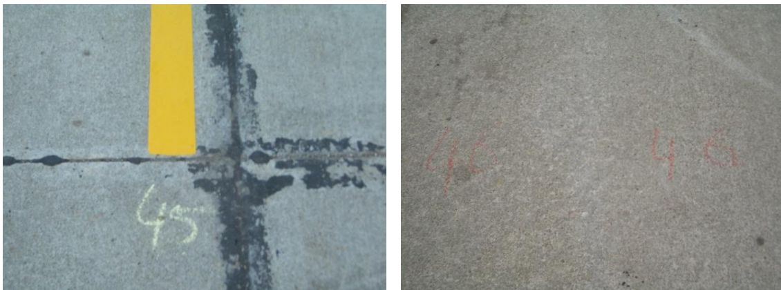
Figure 6.4 Concrete pavement condition before (left) and after (right) tape has been removed by water blasting
