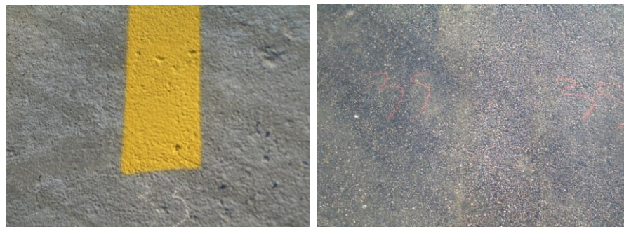
Figure 6.19 Asphalt pavement condition before (left) and after (right) paint has been removed by chemicals
