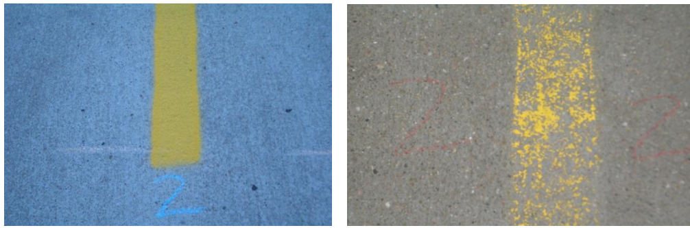
Figure 6.7 Concrete pavement condition before (left) and after (right) 10 mils water-based paint has been removed by dry ice blasting
