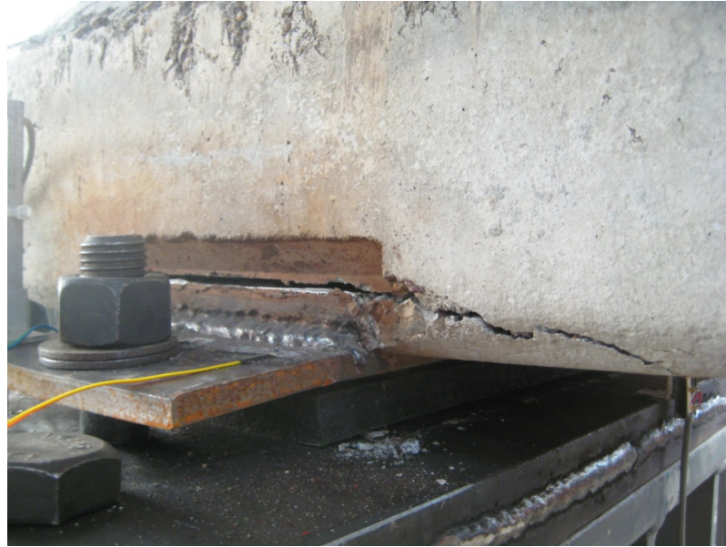
Figure 22: Cracking of specimen HS-1.
