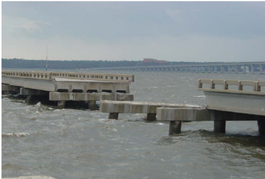
Figure 1: Example of damage at Escambia Bay, FL, after Hurricane Ivan (Courtesy W. Nickas).
