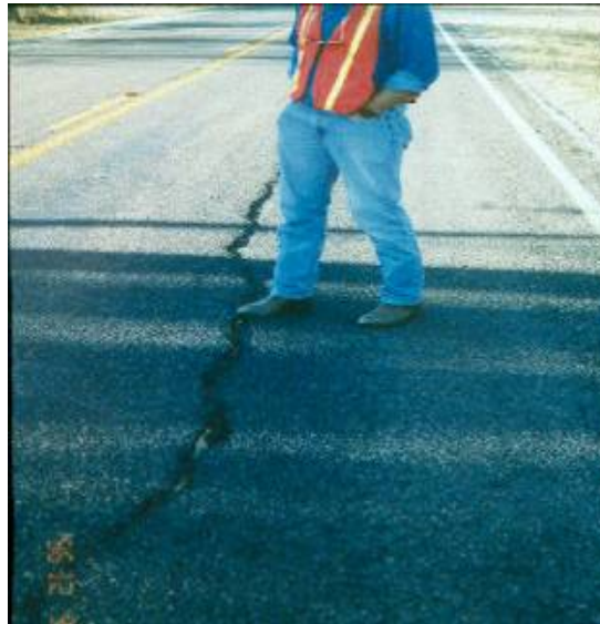
Figure 4.1. Longitudinal Cracking on FDR Projects.
