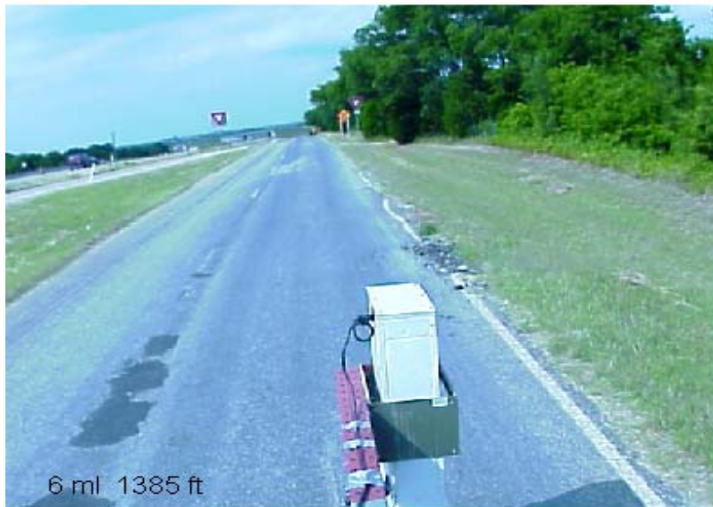
Figure 1.11. Distressed Condition of IH 35 Frontage Road in Dallas District.
