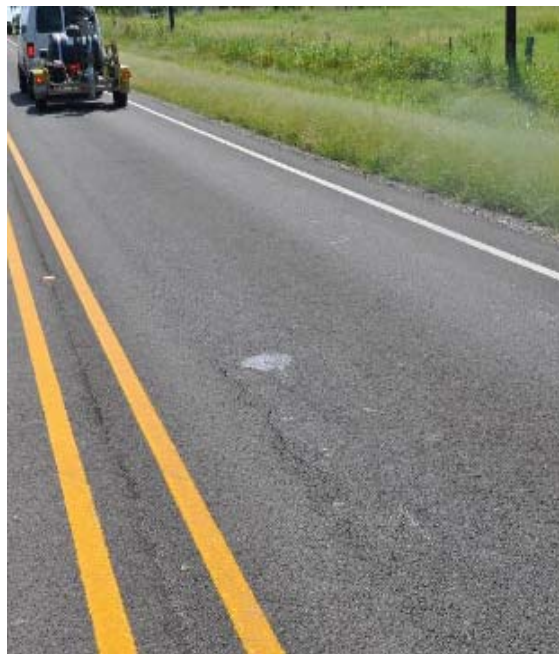
Figure 4.7. Alligator Cracking and Rutting a Few Months after Construction.
