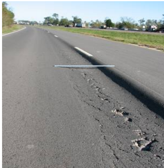
Figure 4.6. Failure in One Wheel-Path Only.
