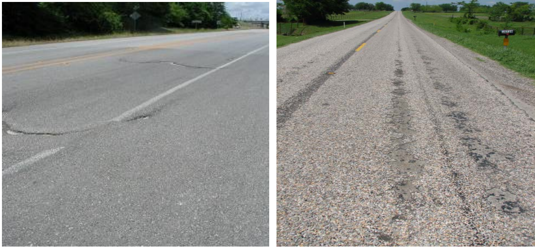
Figure 4.4. HMA Bonding Problems and Seal Coat Pop-Outs over Stabilizer Base.
