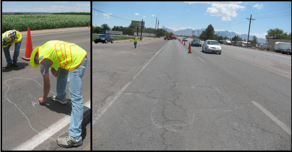
FIGURE 35 Examples of alligator cracking area that is wider than 2 ft and lies outside the limits of the wheel paths. Areas are outlined on the pavement surface
