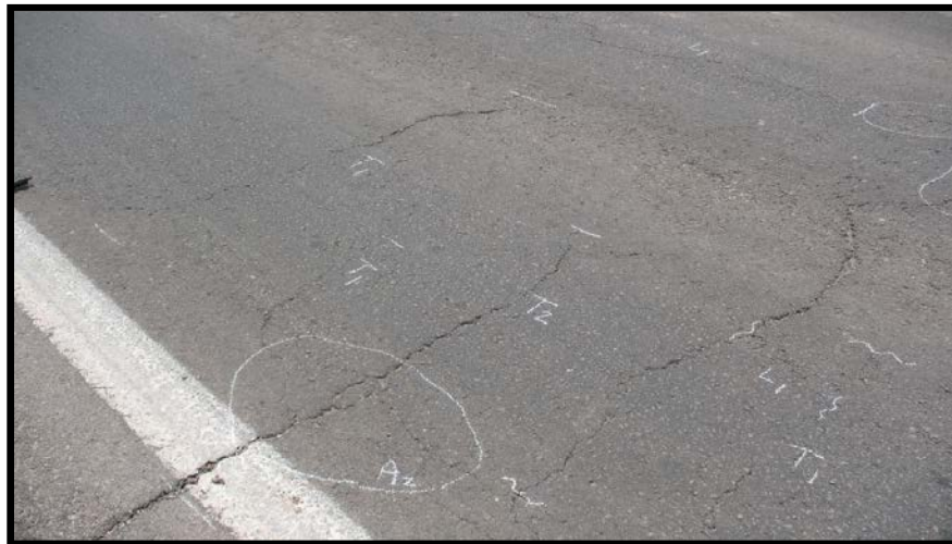
FIGURE 26 Markings on the pavement surface for transverse cracks and alligator cracking in preparation for length and area measurements of these distresses
