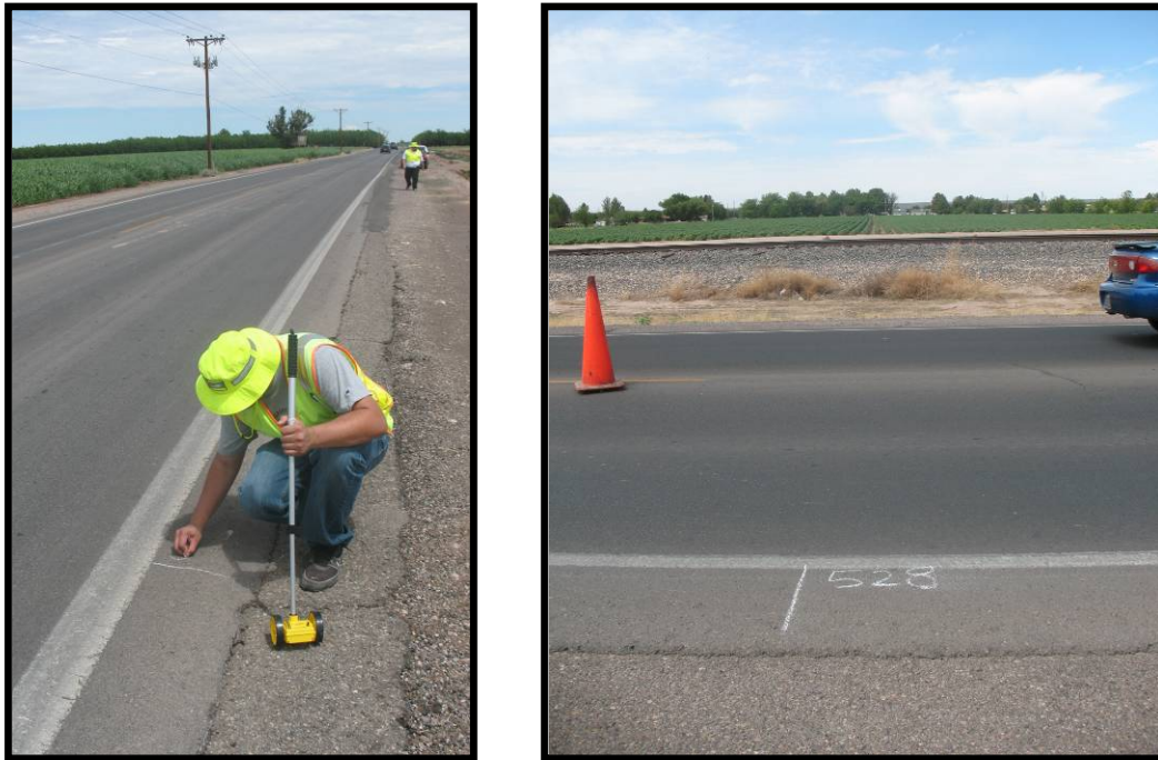
FIGURE 25 A rater marks the start and end of the test section before the field measurements in NM 28
