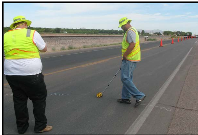
FIGURE 27 A student technician measures the length of transverse cracks while his partner records the data
