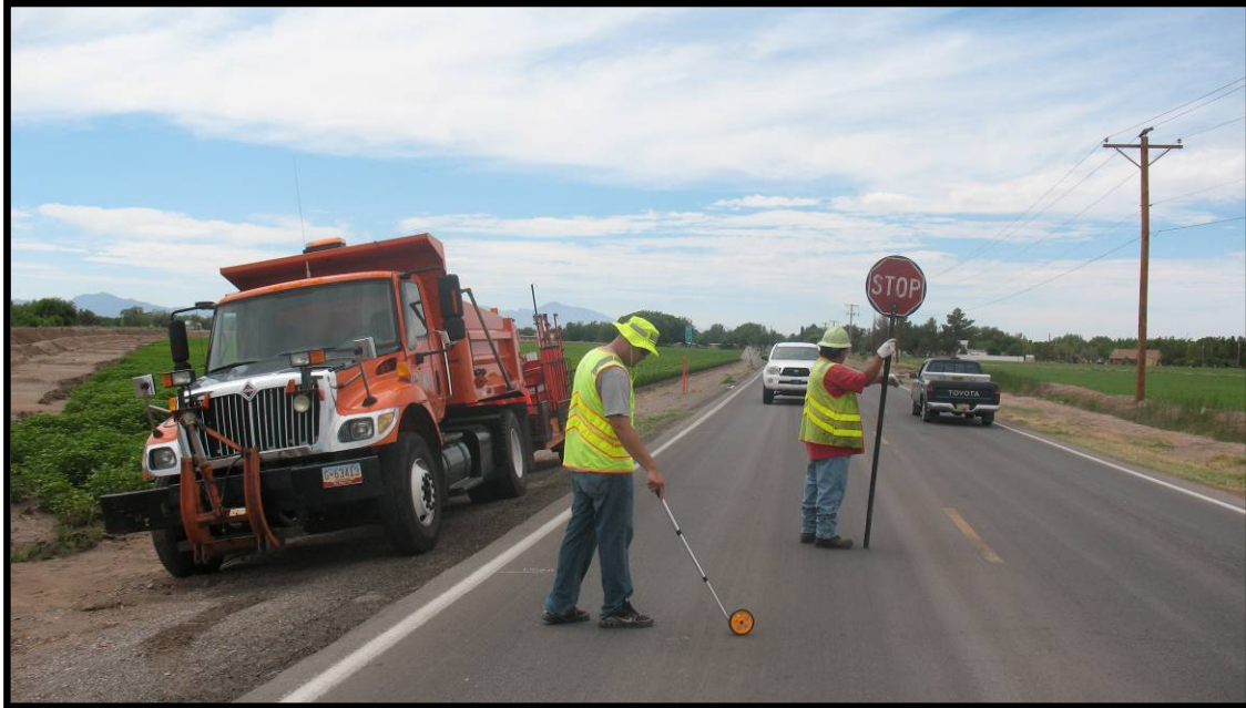
FIGURE 24 The NMDOT District 1 Maintenance Crew of Las Cruces provides traffic control and warning signs during field measurements
