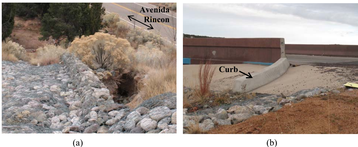
Figure 15. Reconstructed riprap rundown in highway NM 599 (2007): (a) extensive erosion (downslope view); (b) flume with curb added.
