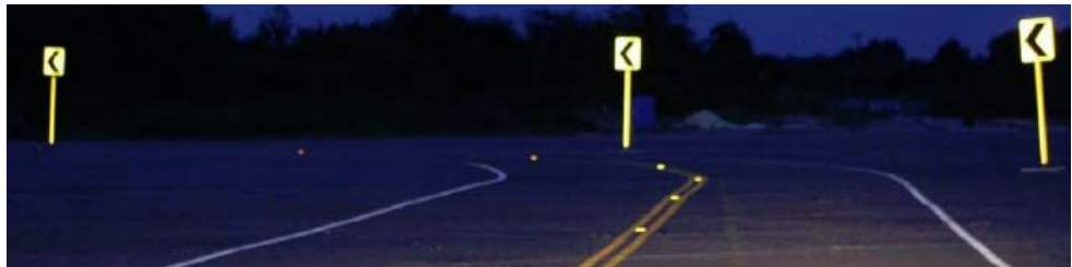
Full Post Chevron (adding reflectorized strip to post) --- chevron is already in place, reflector strip is added to post (image source: TTI)
