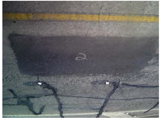
Figure 60. Patch 2 on Site IH410Fr-1.
