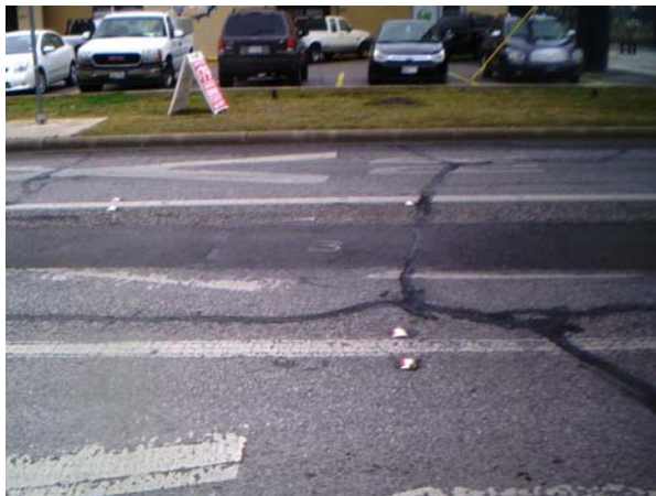
Figure 61. Patch 3 on Site IH410Fr-2.
