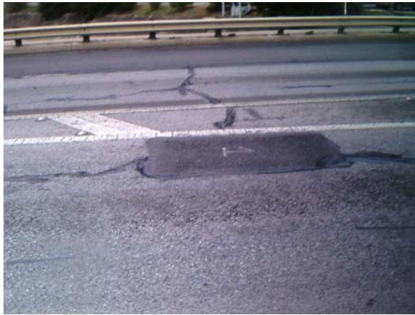
Figure 59. Patch 1 on Site IH410Fr-1.
