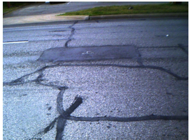
Figure 62. Patch 4 on Site IH410Fr-2.
