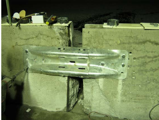
Figure 17: Maine repair of a PCB joint experiencing ASR expansion (Peabody, 2011)
