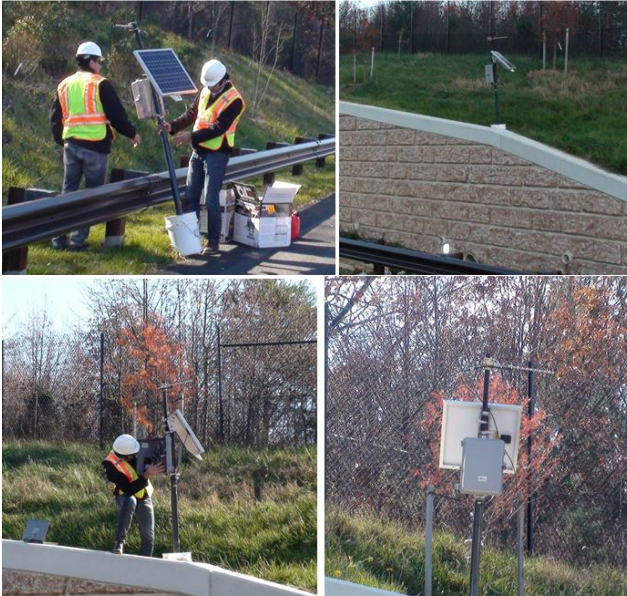
Figure 24. Roadside data collector installation on Inter County Connector test site
