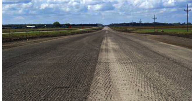
The asphalt removed from this milled road surface contributed to the many tons of asphalt reclaimed each year during road repair operations.
