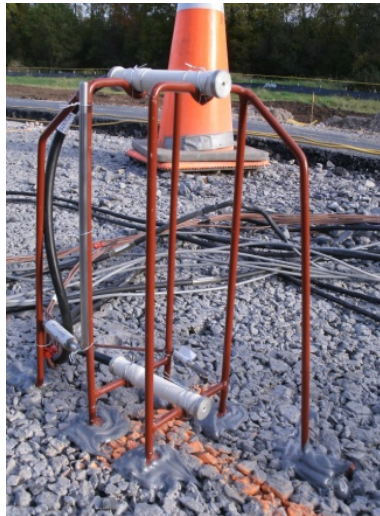
Figure 4 Paired KM strain gauges and supporting metal chair
