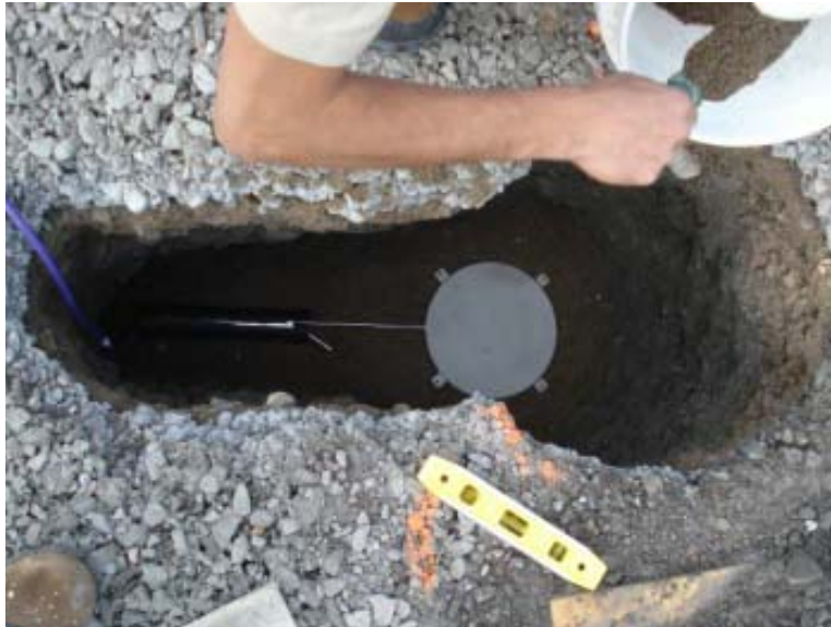
Figure 7 Earth pressure cell beneath the DGAB layer
