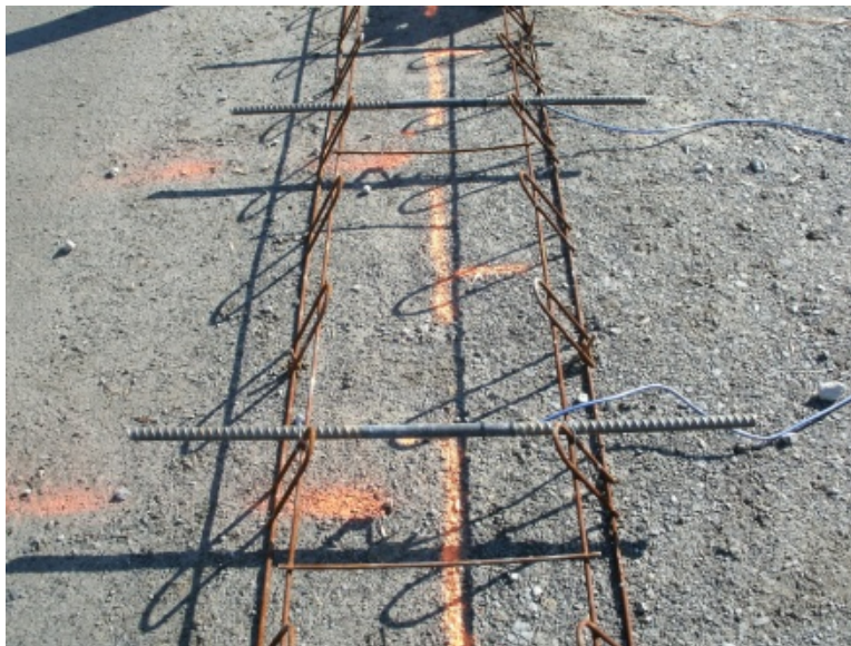
Figure 5 Geocon vibrating wire strain gauge tie bars placed at longitudinal joint
