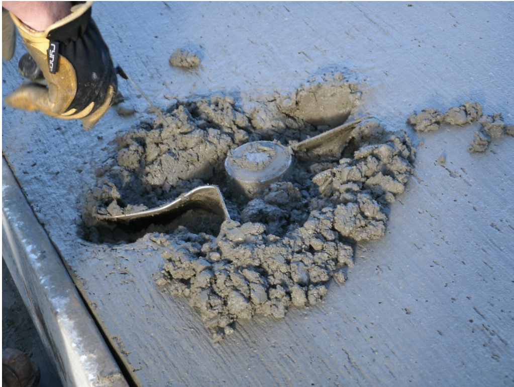
Figure 11 LVDT 2 in Section 2 after paver struck metal box
