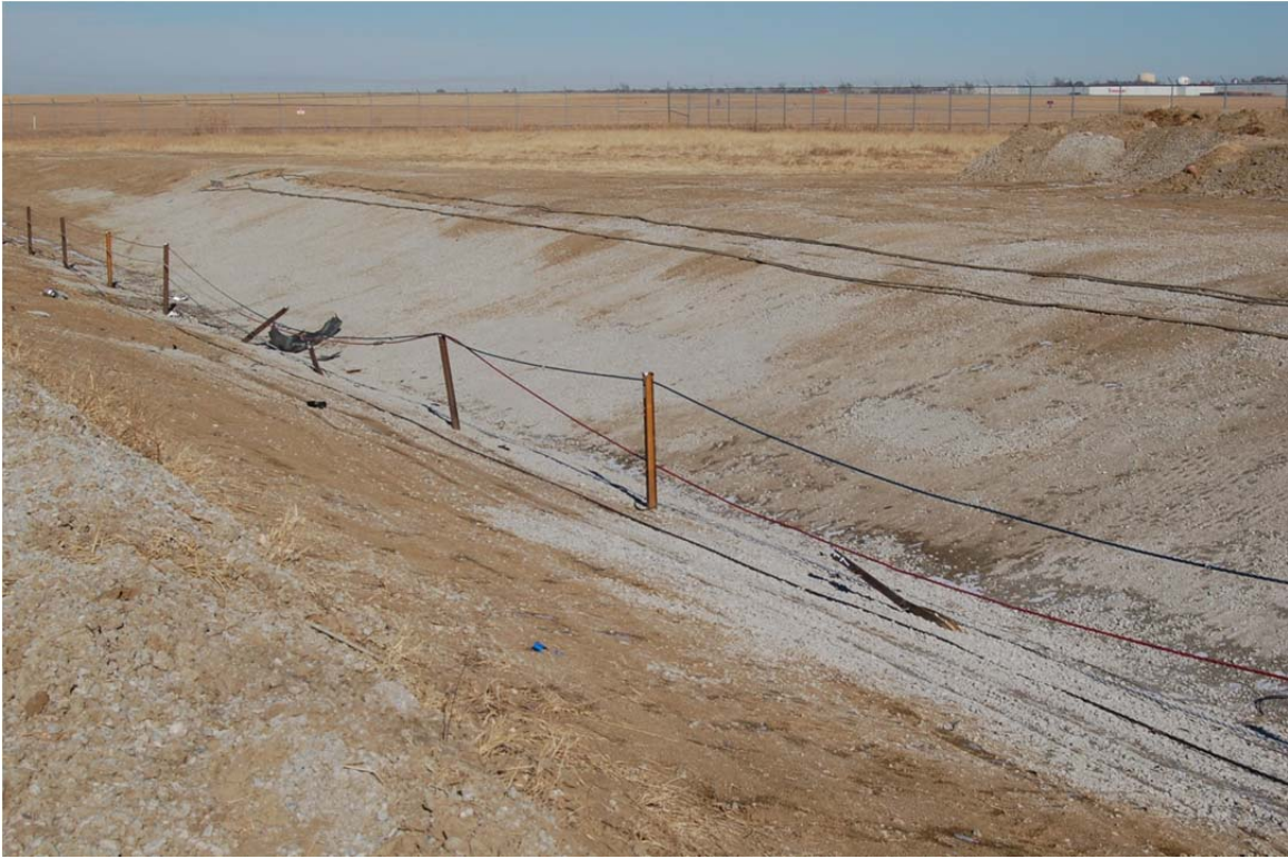
Figure 42. System Damage, Test No. 4CMB-4
