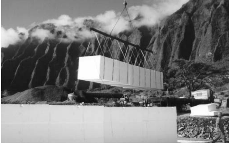
Figure 2.72. Emergency Ramp and High Embankment Constructed Using the EPS Geofram at Kaneohe Interchange in Oahu, Hawaii.
