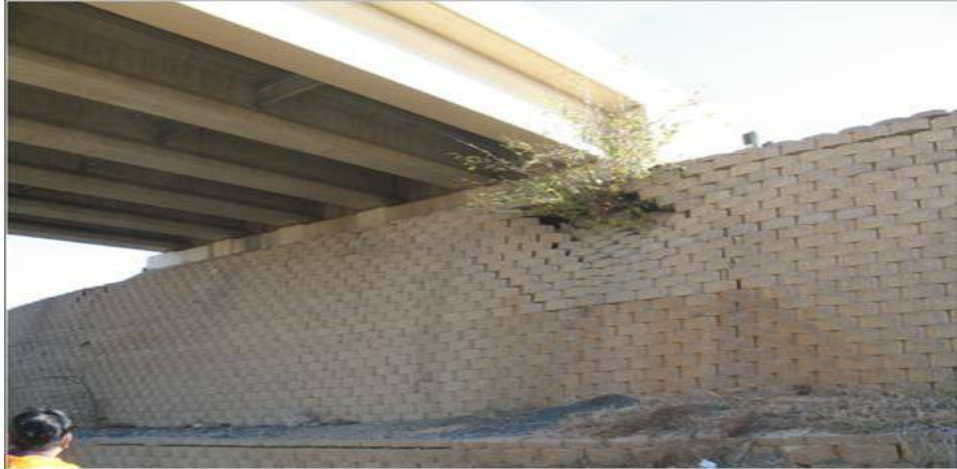
Figure 9.15. Failure of the Modular Block Wall.
