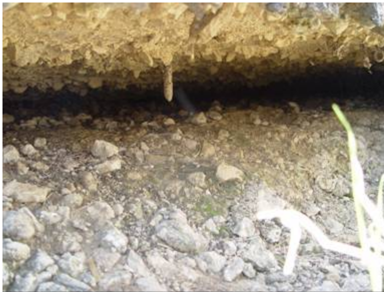
Figure 9.5. Closer View of the Void.
