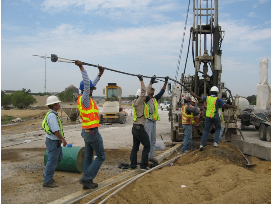
Figure 6.30. Placement of the Assembled Rods and Reference Head into the Drilled Hole.
