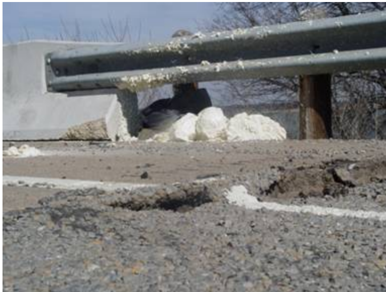
Figure 9.11. Another View of the Pavement Differential of the Approach Slab.
