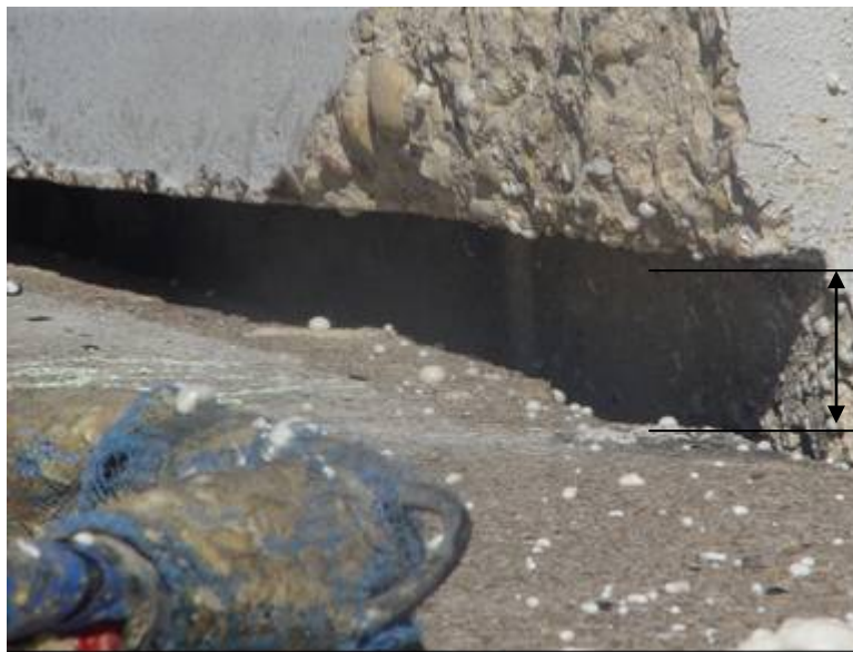
Figure 9.3. Settlement of the Approach Slab.
