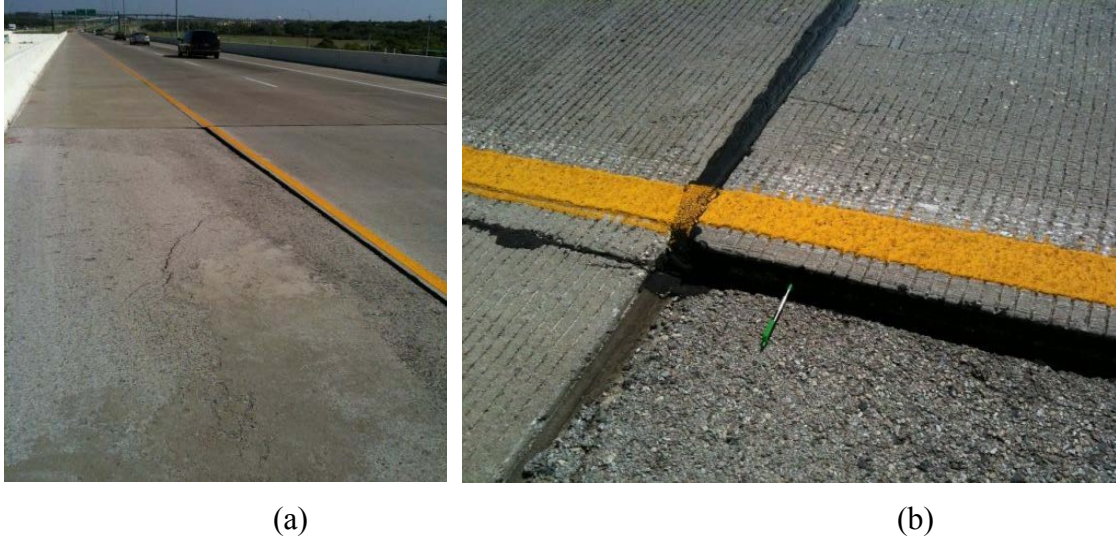
Figure 7.25. Opening Observed between the Highway Mainlanes Pavement and Its Shoulder.
