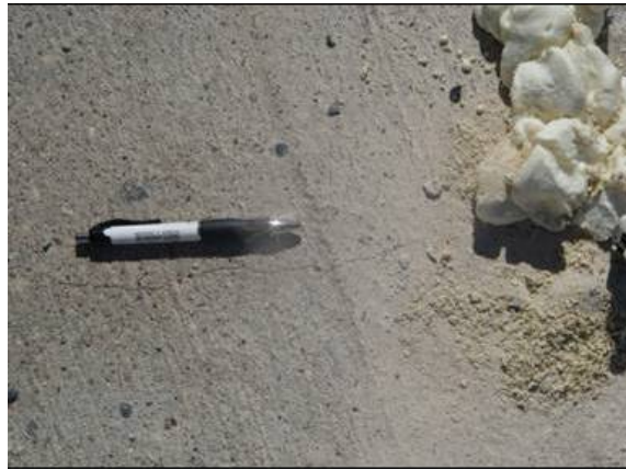
Figure 2.68. Hairline Crack Observed on the Approach Slab during the Urethane Foam Injection.
