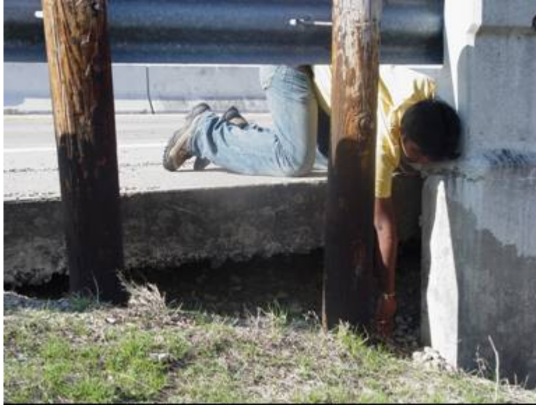
Figure 9.4. Void Formation Adjacent to the Abutment.
