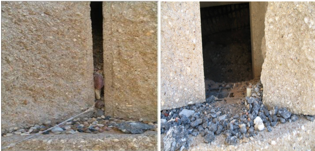
Figure 9.16. Erosion of the Soil under the Slab.
