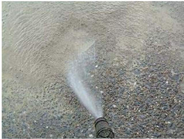
Figure 3.1. Surface mortar being washed away to expose aggregates
