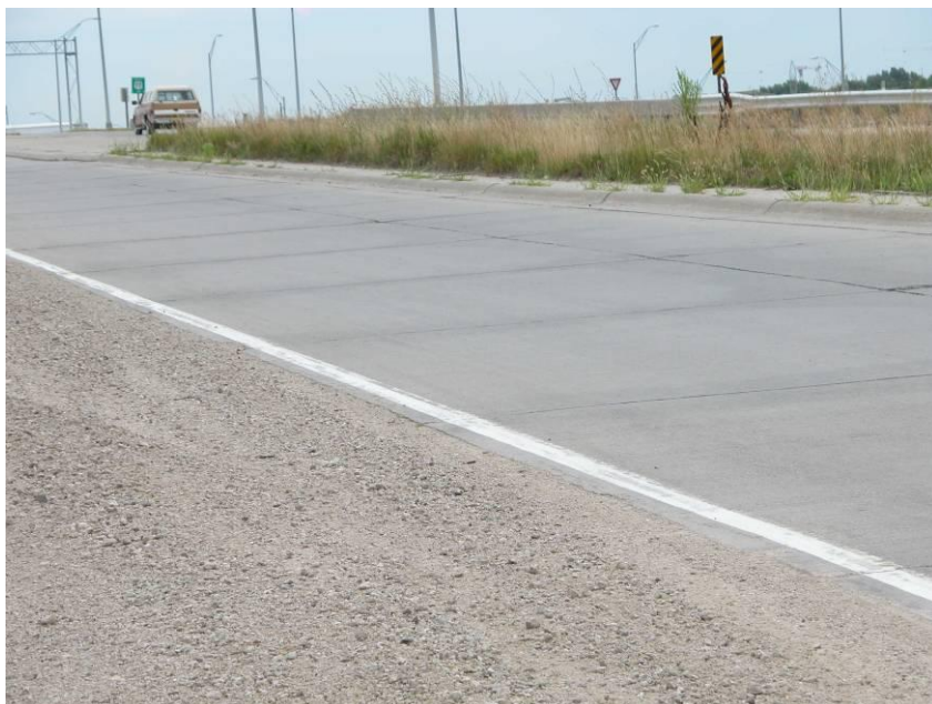
Staining of Joints
