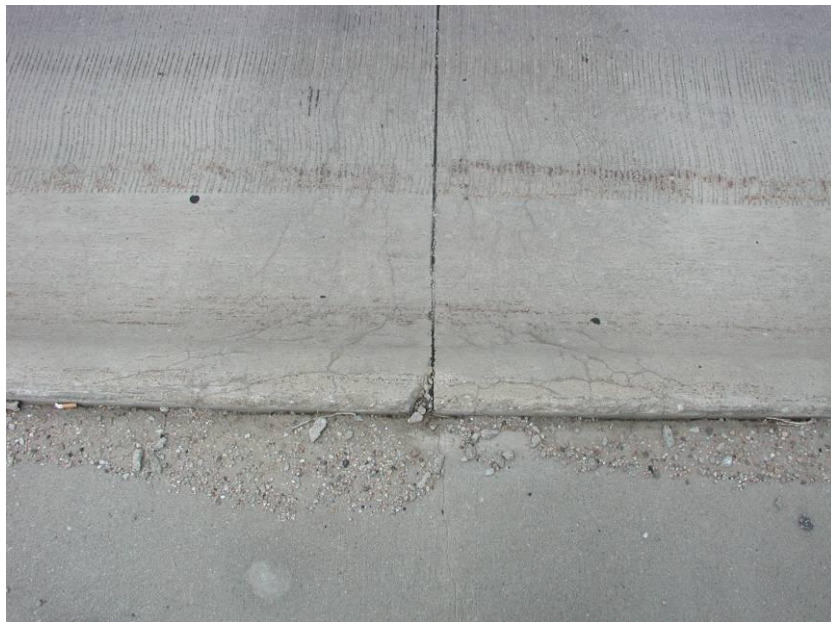
Cracking Running Adjacent to Free Edges and Joints
