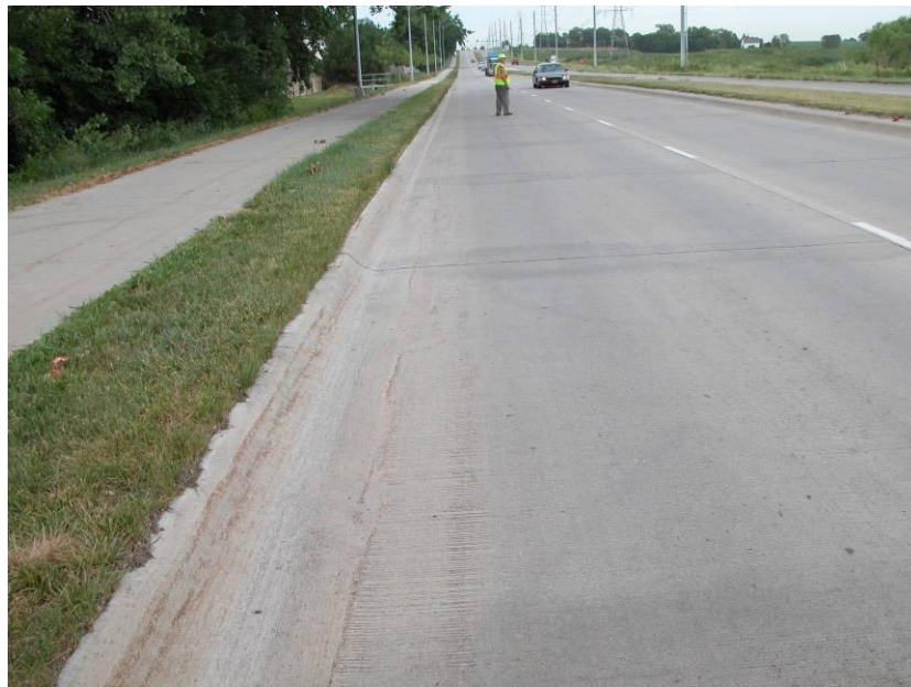
Staining of Transverse Joints
