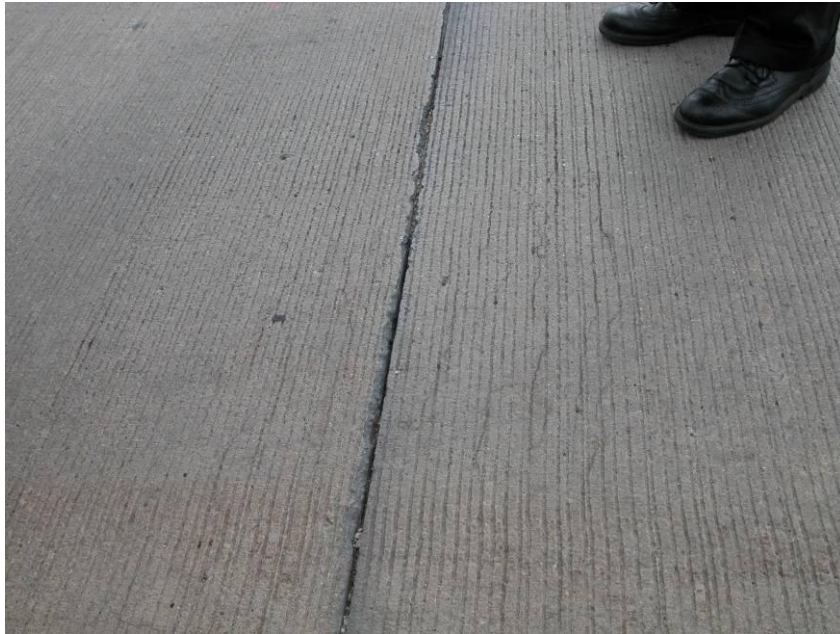
Cracking Parallel to the Joint
