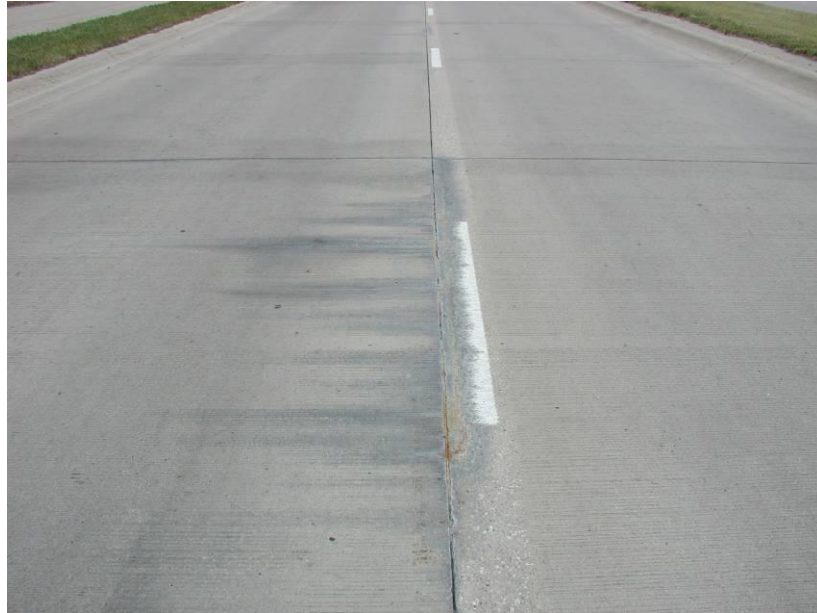
Staining of Transverse and Longitudinal Joints
