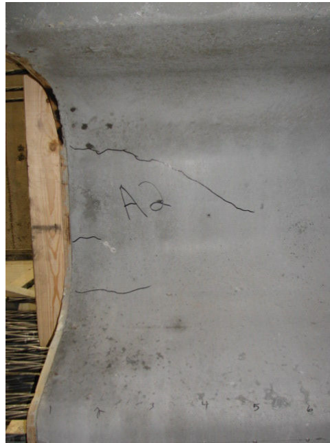
Figure 2.7.2: A2 end zone cracking
