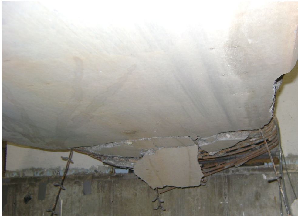
Figure 4.6.2.2: Failure near diaphragm
