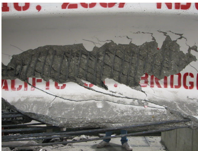
Figure 2.11.4.6: Shear cracking in web and split flange
