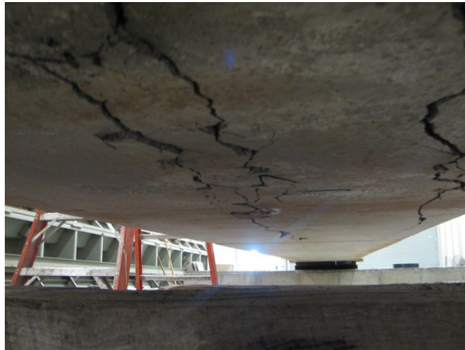
Figure 2.11.4.12: Longitudinal flange cracking
