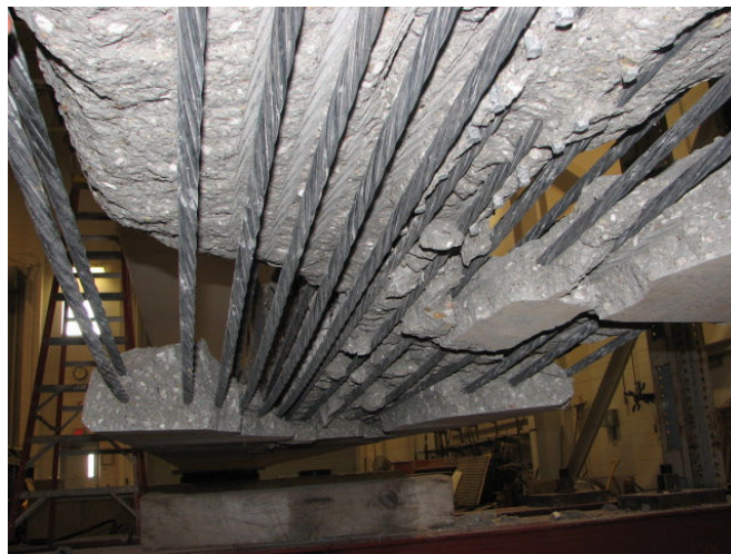
Figure 2.11.4.13: Loose strands after failure
