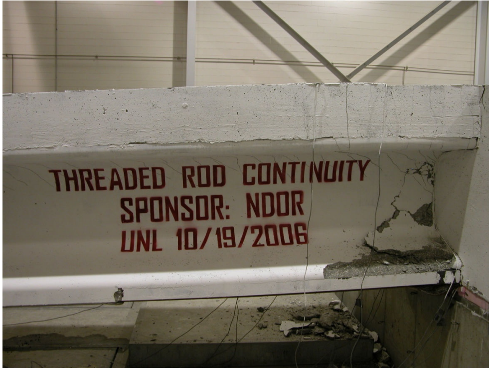
Figure 3.3.27: Specimen Failure at 382 kips
