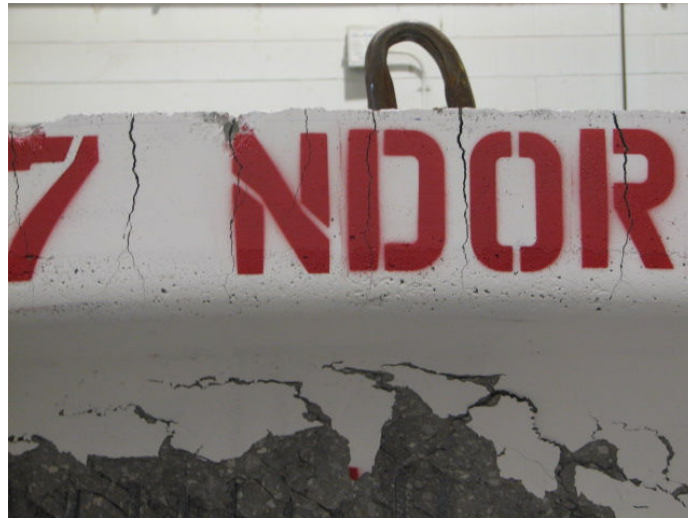
Figure 2.11.4.9: Tensile deck cracking
