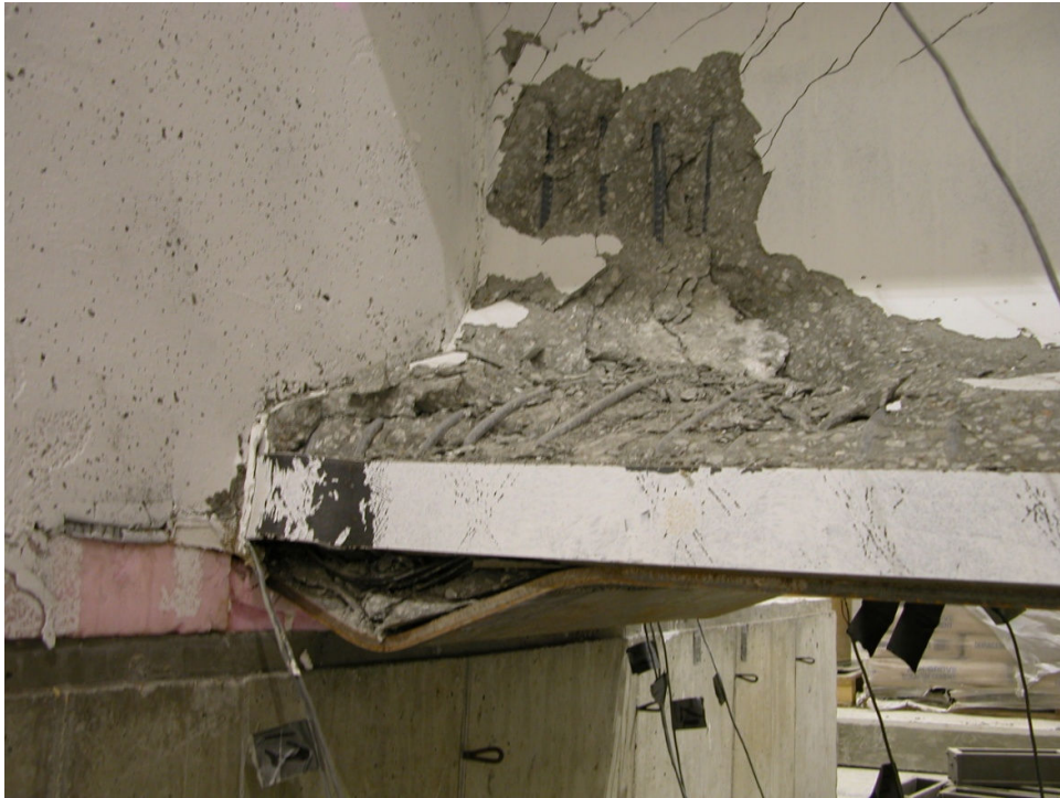
Figure 3.3.28: Shoe Plate Buckled at the Face of Diaphragm
