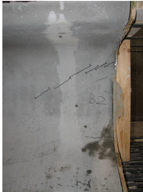
Figure 2.7.4: B2 end zone cracking
