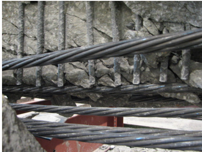
Figure 2.11.4.10: Shear reinforcement non-bent in bottom flange
