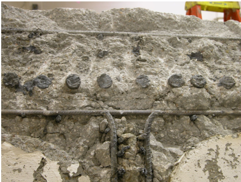
Figure 3.3.30: No Slippage between TR and the Concrete around them
