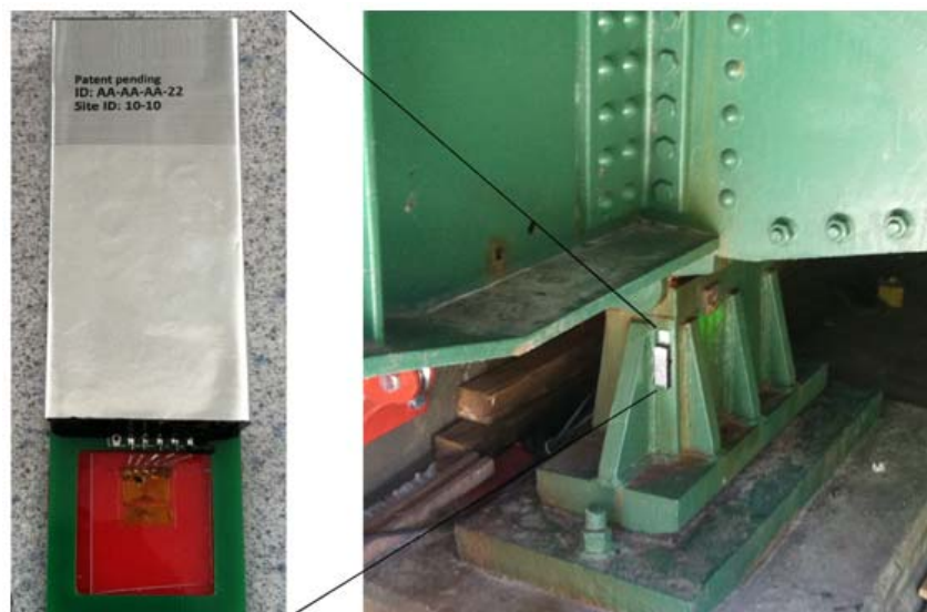
Figure 1: A SenSpot (left) and installed sensor on a bridge bearing (right) for tilt and loading monitoring.
