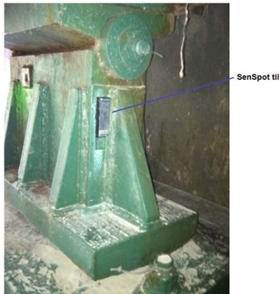
Figure 8: Wireless tilt sensor on a rocker bearing of Northwest Branch Bridge on I-495
