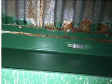
Figure 13: Installed SenSpot strain under the deck of Northwest Branch Bridge on I-495.
