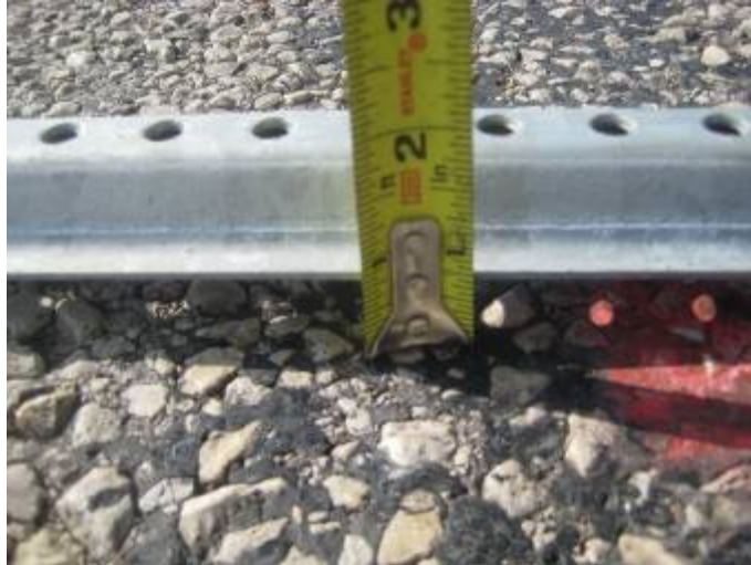
Figure 83. Rutting on FM 2674.
