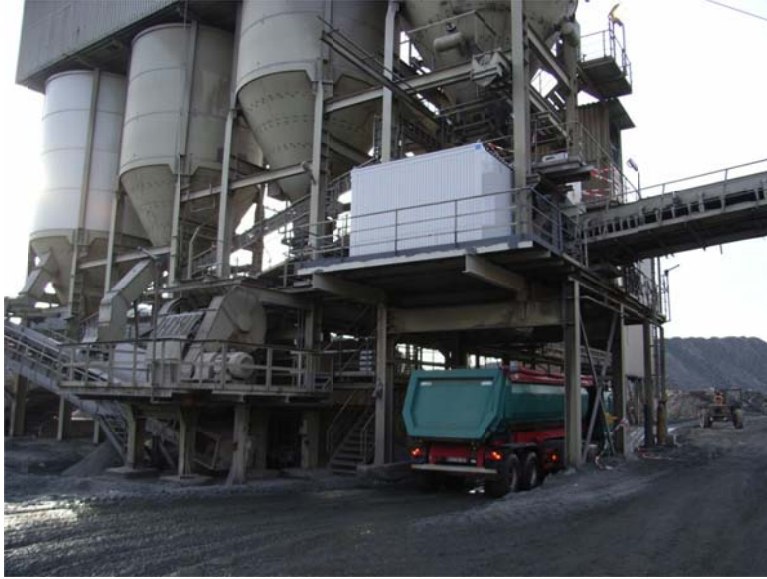
Figure 15 CPA 4-2 Housed in a Container at an Aggregate Crusher
